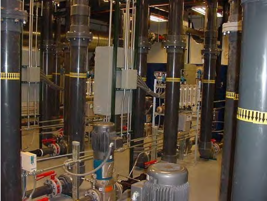
Photo 1. Gelman Ozone/Hydrogen Peroxide Treatment System
