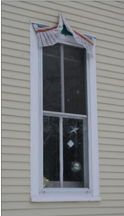
Historic windows should be preserved and maintained. The Historic District Commission will not consider approval of historic window replacement unless window parts are deteriorated beyond repair.
