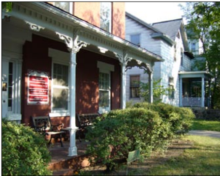
Repair and maintain all porches and do not allow them to deteriorate.
