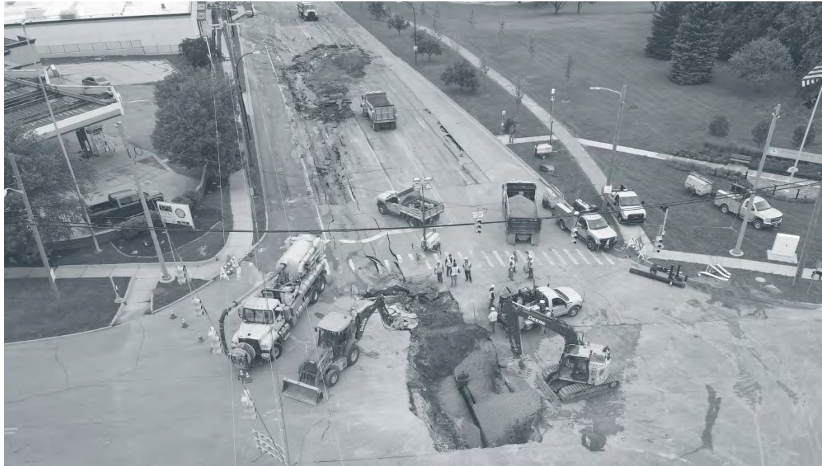
Figure 4-52: June 2021 Water Main Break
