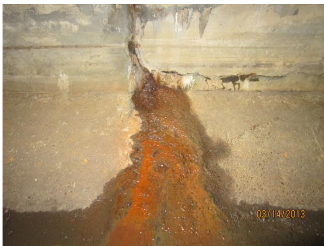
Photo 24 Station 600+20: joint leak
