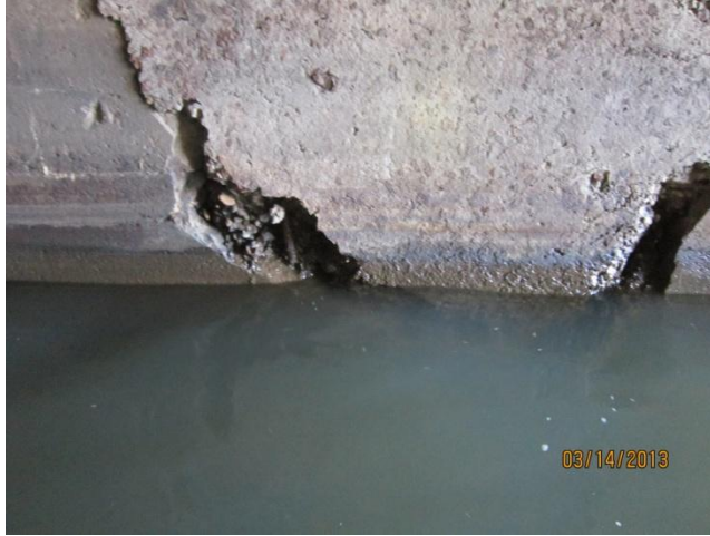
Photo 4 Station 100+45: old repair light to medium
