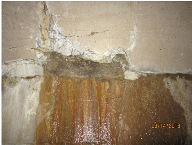
Photo 5 Station 100+65: crack in wall, seam leaking
