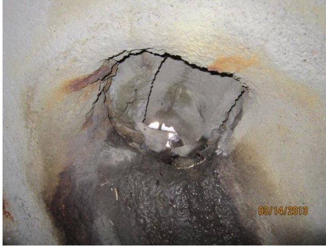
Photo 31 Station 800+20: curb inlet, poor condition
