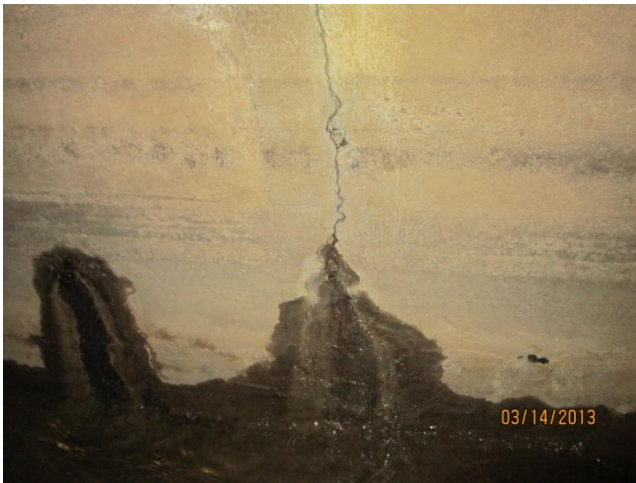
Photo 17 Station 300+5: seam leak, crack in grout
