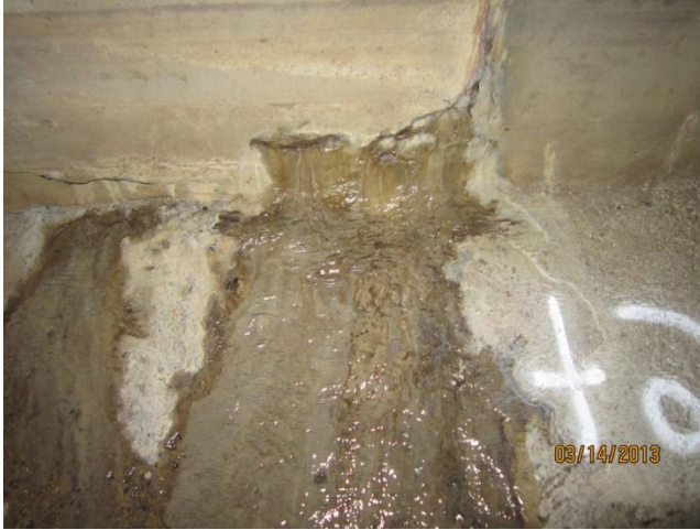
Photo 25 Station 600+20: joint leak, crack in grout
