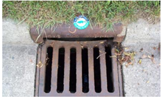
Figure 3 - Example of label embedded in drain grates through Adopt-a-Drain program
