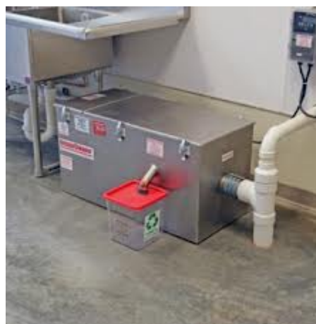
Figure 13: Typical Grease Accumulator near the kitchen sink
