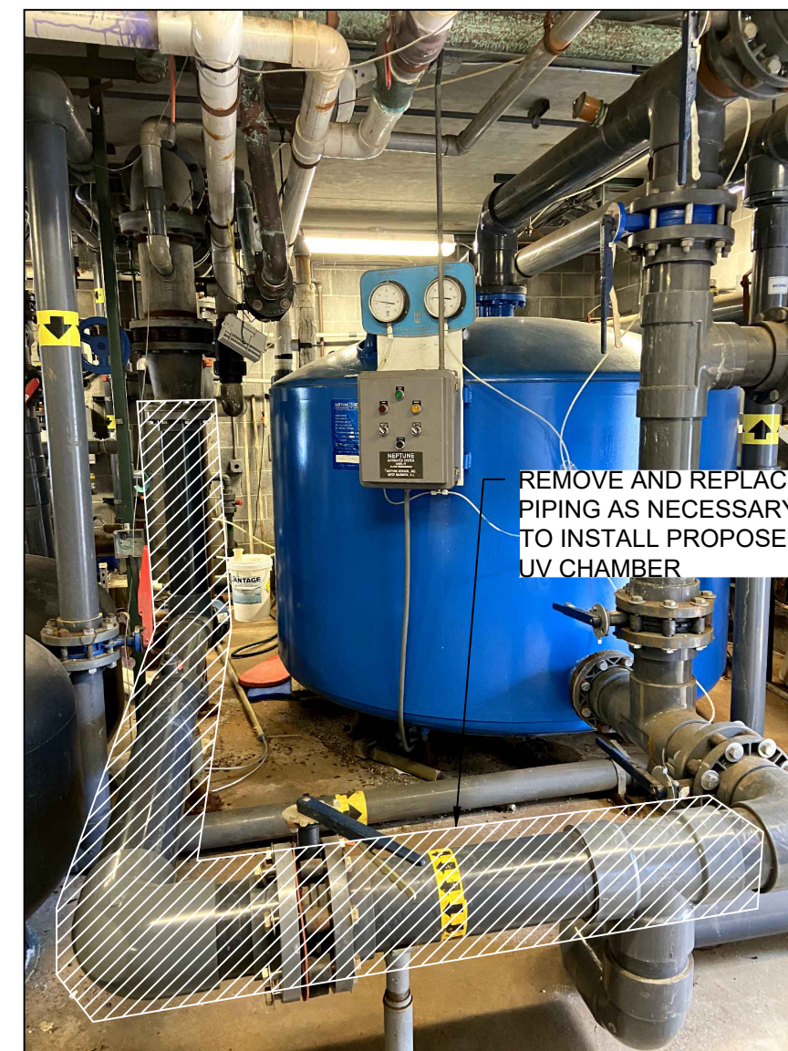
EXISTING MAIN POOL DISCHARGE PIPING
