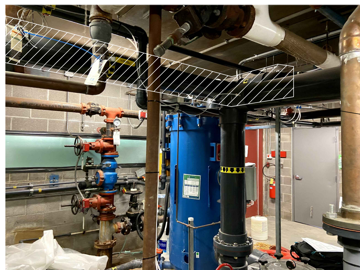
EXISTING POOL DISCHARGE PIPING
