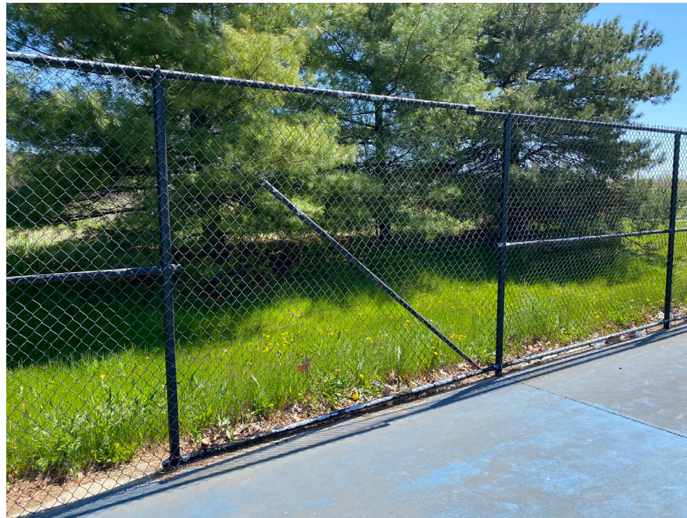
FENCE ALONG BASKETBALL COURT TO REMAIN - TAKE DOWN AS NECESSARY DURING CONSTRUCTION.
