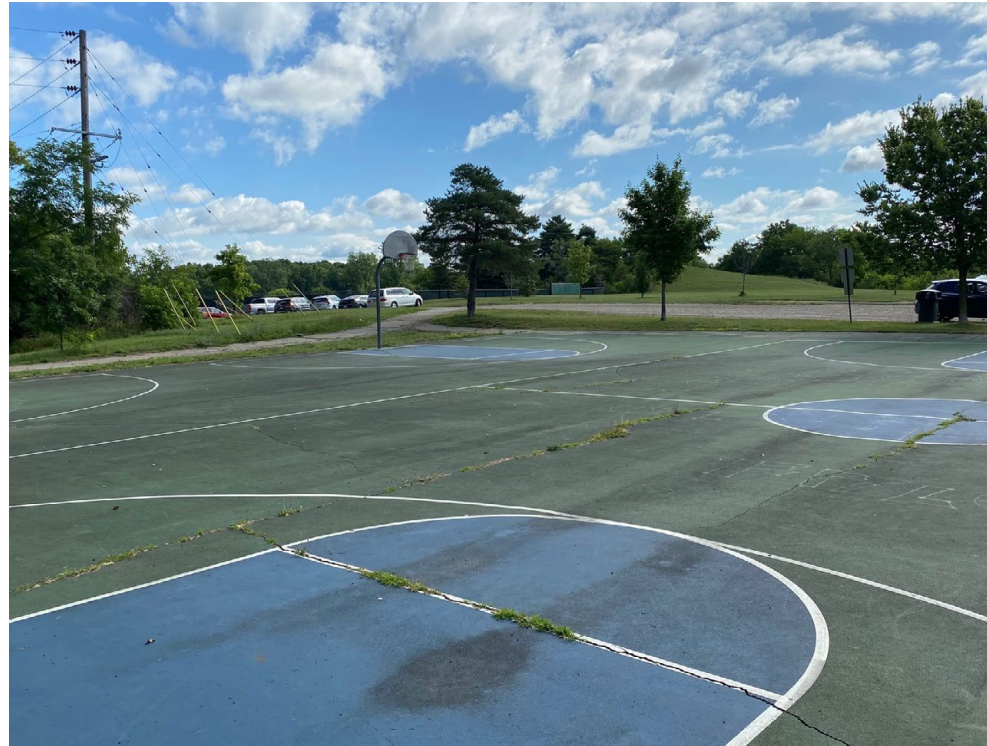
NEW STRIPING AND COATINGS TO MATCH EXISTING COURT LAYOUT (ONE FULL COURT, TWO HALF COURTS)
