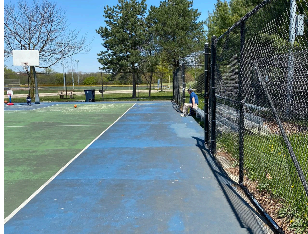
FENCE ALONG BASKETBALL COURT TO REMAIN - TAKE DOWN AS NECESSARY DURING CONSTRUCTION.
