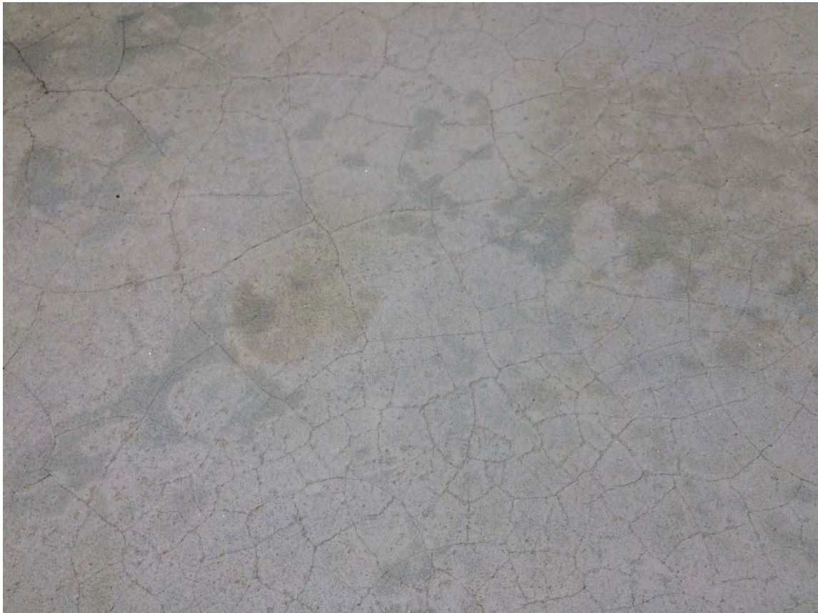
Delaminating Marcite in wading pool
