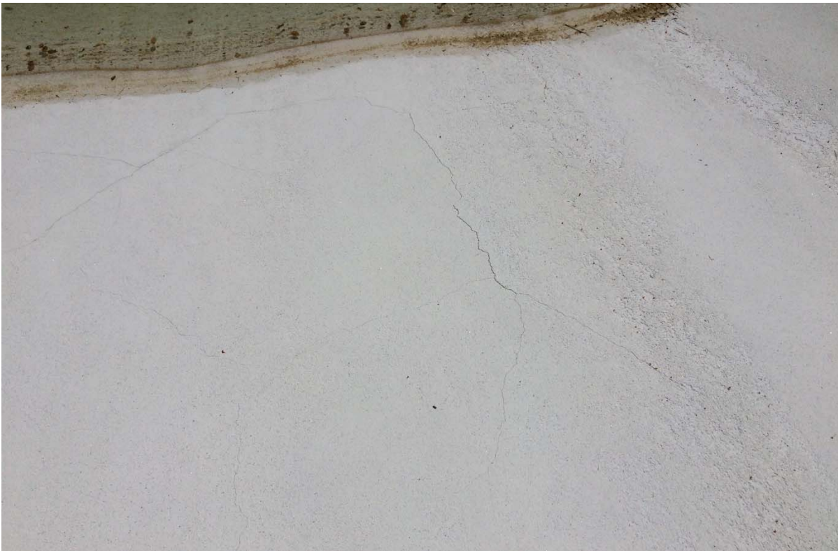
Delaminating Marcite on sloped floor of the deep pool
