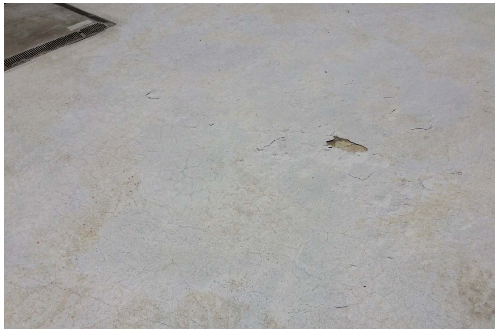
Delaminating Marcite in wading pool
