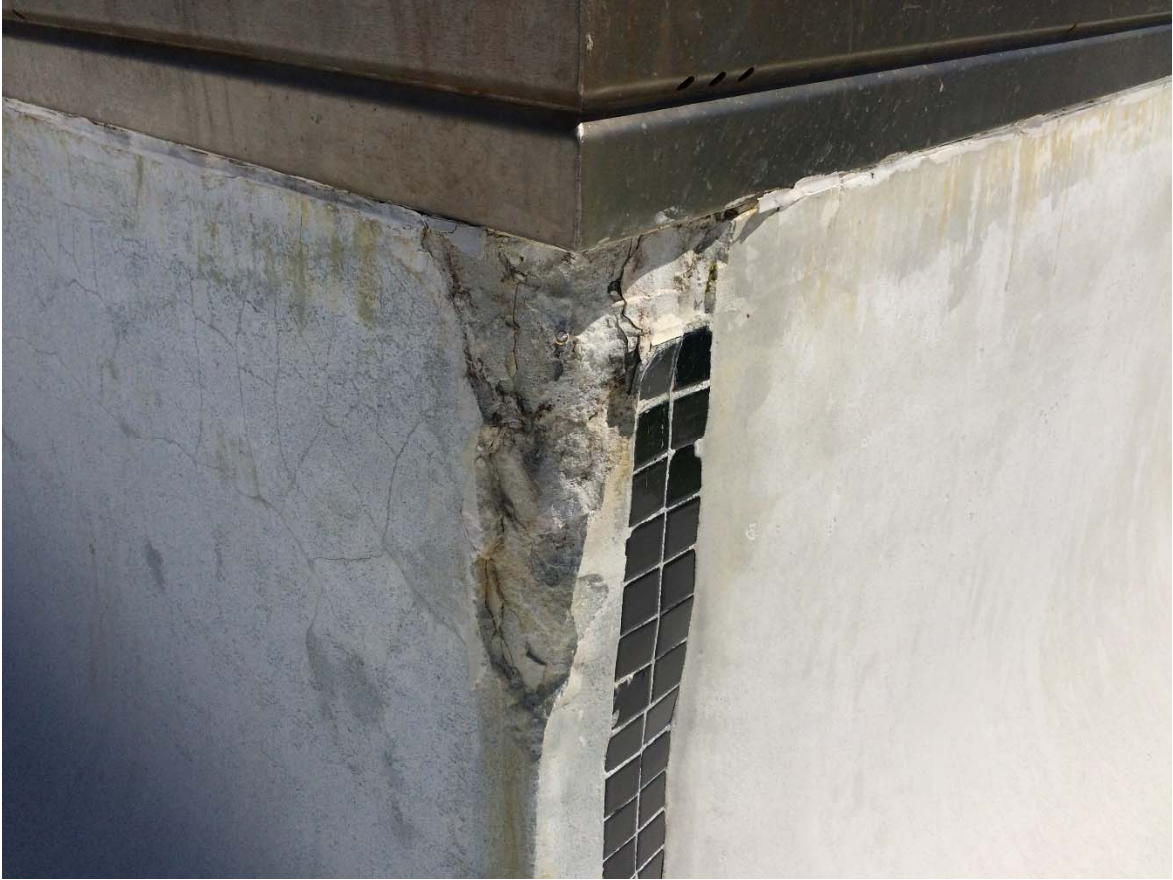
Spalling concrete on NE corner of deep pool
