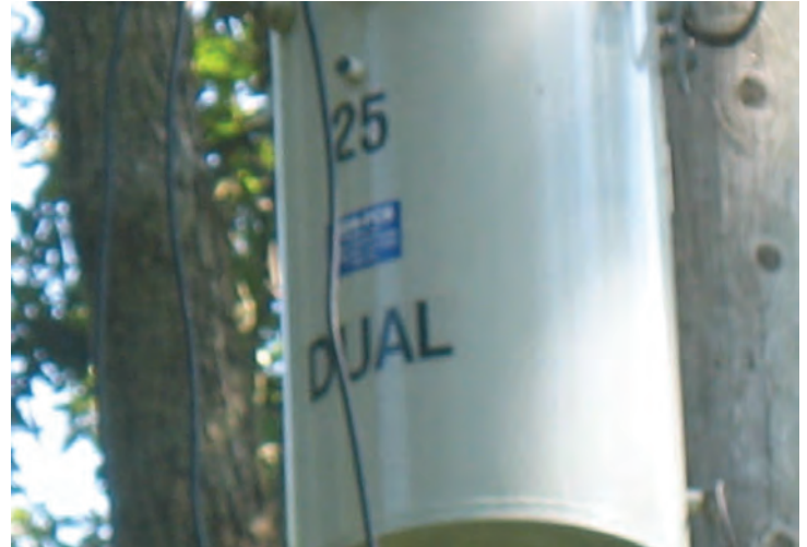
Viewing the non-PCB containing label located on the previously mentioned pole-mounted transformer.
