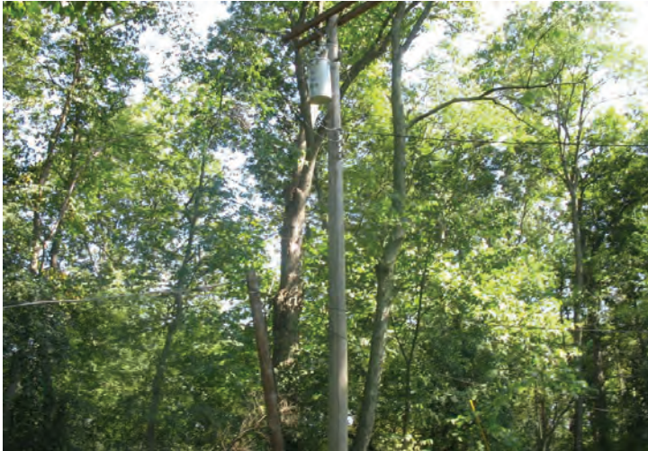
Facing east from the east side of the house viewing a single pole-mounted transformer.
