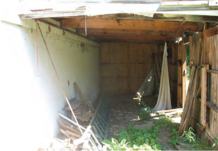
Facing east viewing an exterior storage area located adjacent to the house.
