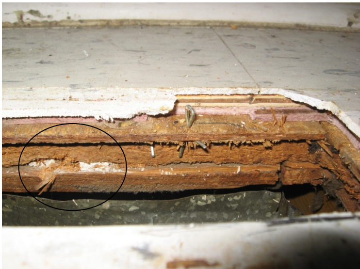
Photo 2. Asbestos-containing floor tile observed in apartment unit 3451 second floor bedroom sub-floor layers. Observed by removing floor vent. Similar floor tile was not observed in any of the other units.
