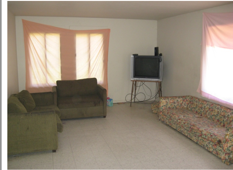
Photo 1. Example of apartment unit drywall with asbestos-containing joint compound.
