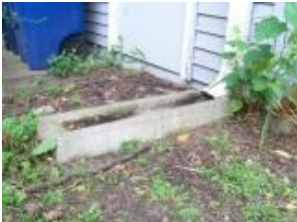
Photo #9: Ground slopes toward the building. Moisture will have a harder time flowing away.
