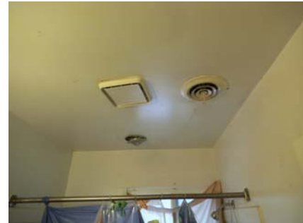
Loose fixtures at bathroom ceiling creating air pathways
