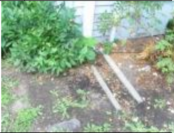
Photo #11: Plants touching and/or overhanging the building should be trimmed.
