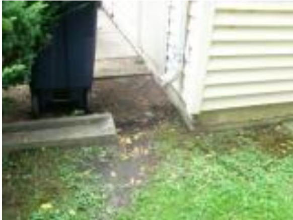
Photo #13: Concrete downspout should be moved closer to building to allow water to flow away.
