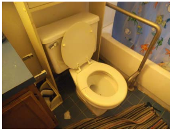
Photo 10: Standard toilet in bathrooms
