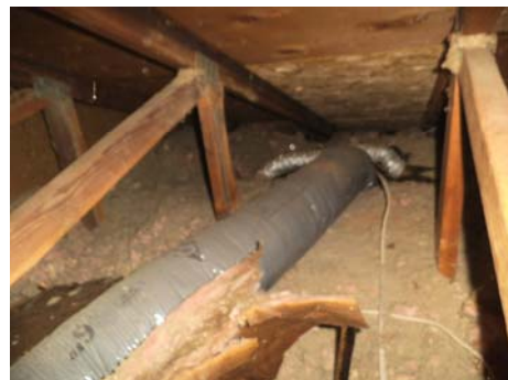
Bath exhaust vent connection to outside should be verified
