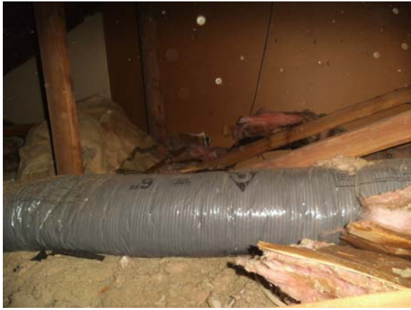
Photo 15: Supply ducting to ceiling registers
