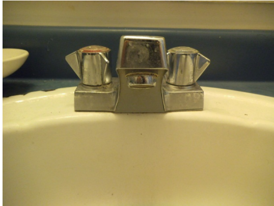
Photo 8: Bathroom faucet with aerator
