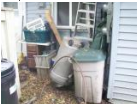
Photo #5: Clutter can hold moisture against the building and provide harborage.
