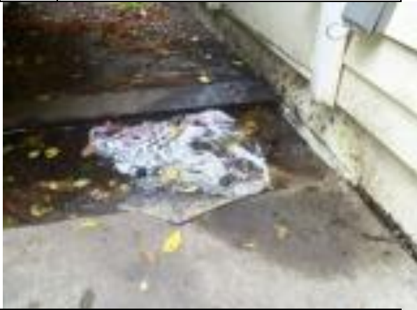
Photo #17: Downspout missing bottom.
