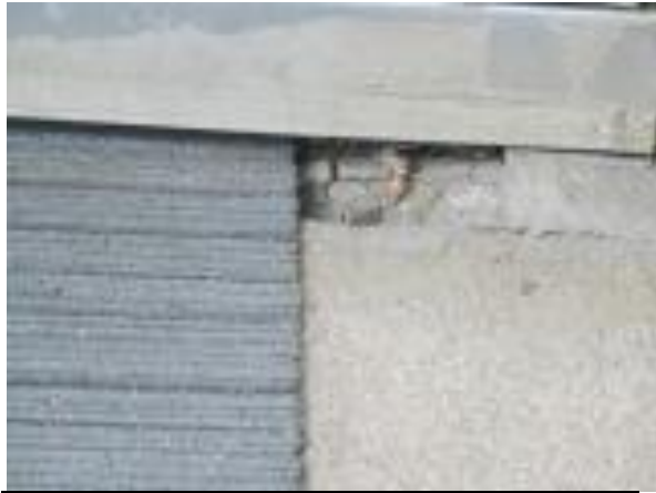
Photo #19: Potential entry point for pests.
