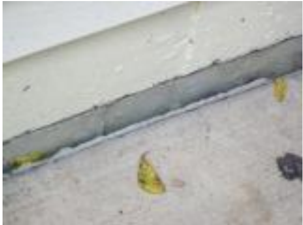
Photo #14: Expansion joint between sidewalk and building should be sealed.
