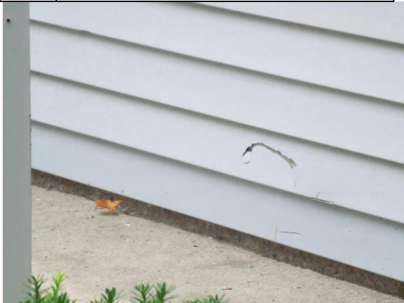
Photo #3: Hole In siding, entry point for pests
