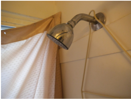
Photo 9: Typical bathroom showerhead
