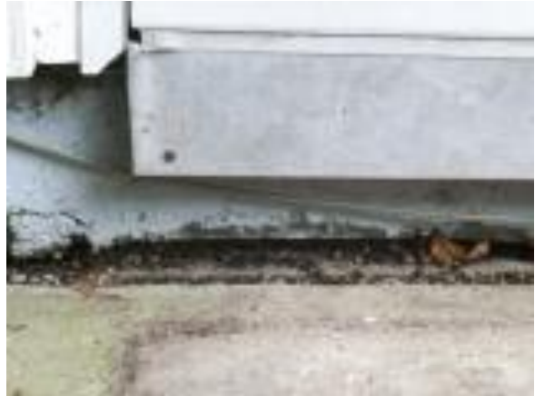
Photo #8: Gap under door potential entry point for pests
