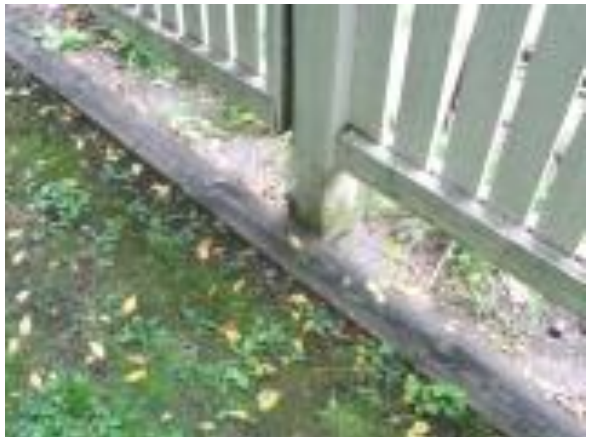
Photo #16: Wood/soil contact is attractive to termites. Railroad ties should be replaced with non-wood alternative.
