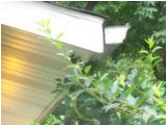
Photo #15: Branches touching roofline should be trimmed
