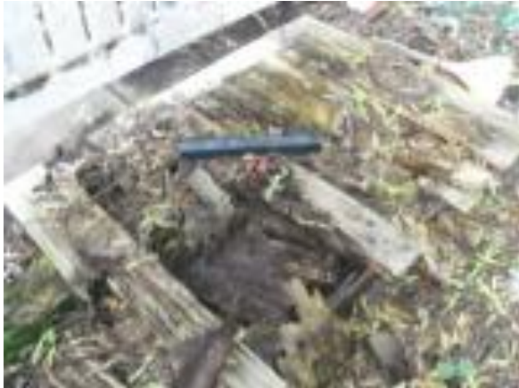
Photo #7: Wood/Soil contact is attractive to termites which have been an issue in the past
