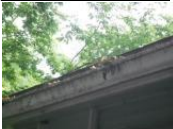
Photo #4: Clogged Gutters can create a moisture issue
