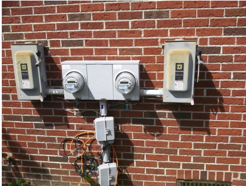
PHOTOGRAPH NO. 7: ELECTRICAL DIS-CONNECT LOCATED BY METER
