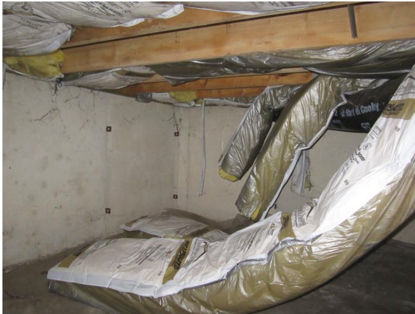
PHOTOGRAPH NO. 14: EXAMPLE OF DROPPED INSULATION IN CRAWL SPACE
