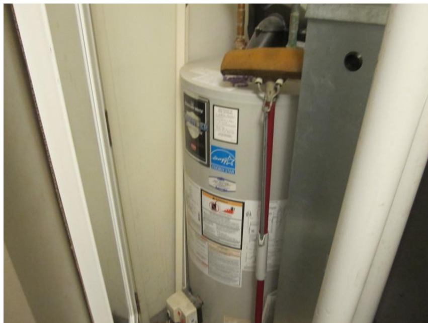
PHOTOGRAPH NO. 8 VIEW OF HOT WATER HEATER IN UNIT
