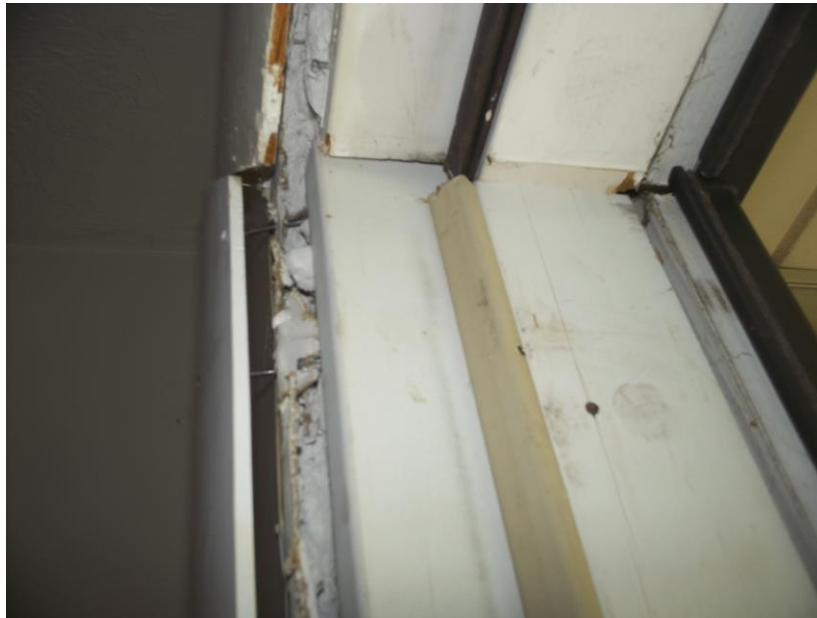
PHOTOGRAPH NO. 6: ISSUES AT ENTRY DOOR
