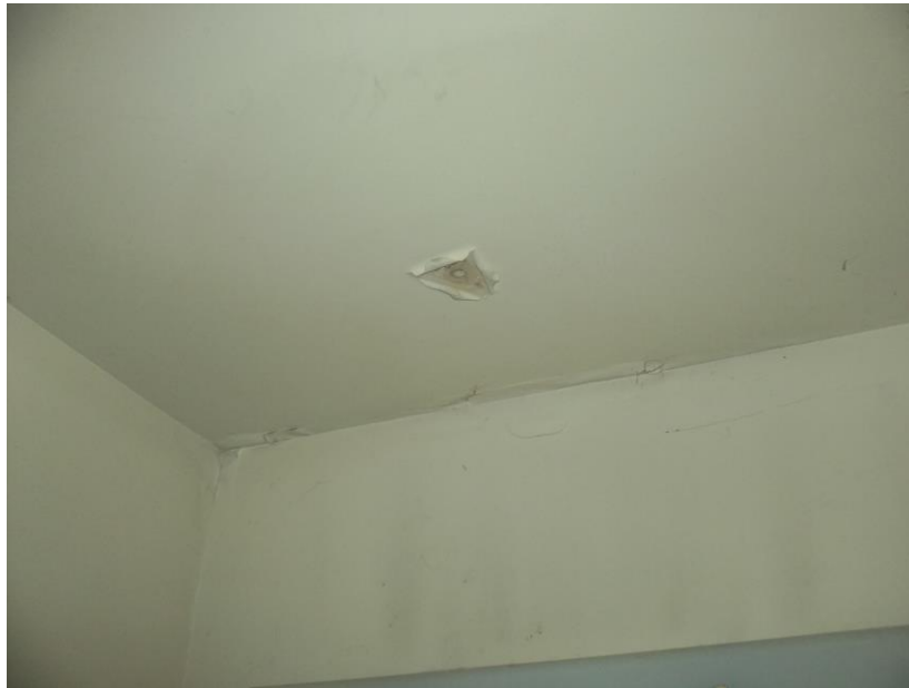
PHOTOGRAPH NO. 12: CEILING MOISTURE PROBLEM (UNIT 2674)
