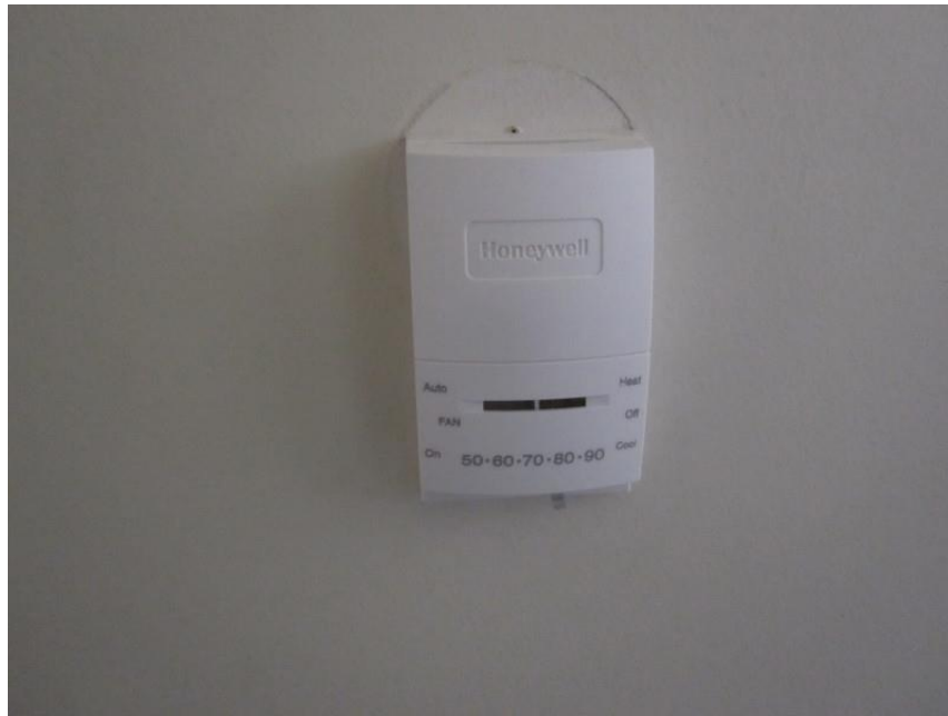
PHOTOGRAPH NO. 15: TYPICAL VIEW OF TENANT UNIT THERMOSTAT
