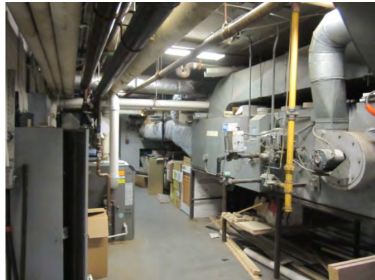
Photo 16: Makeup air unit serving the entire facility
