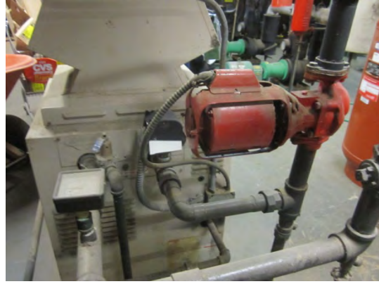
Photo 14: Domestic hot water circulating pump
