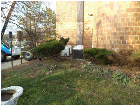
Photo 4: Condensing Units on side of building
