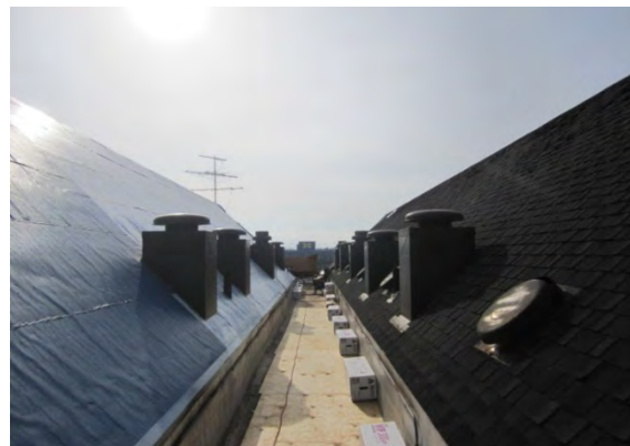
Photo 42: Typical exhaust hoods for unit bathroom
