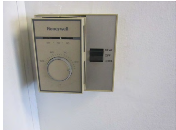
Photo 24: Thermostats for fan coil units
