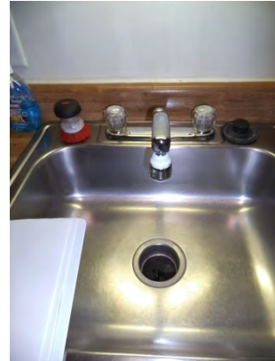
Photo 34: Typical faucet aerator for kitchen sink
