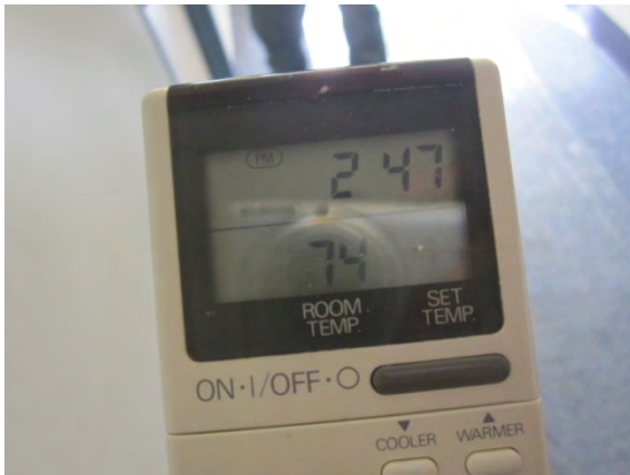
Photo 21: Remote thermostat for Sanyo units
