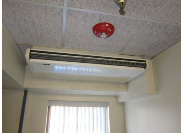
Photo 20: Typical split system at the end of hall
