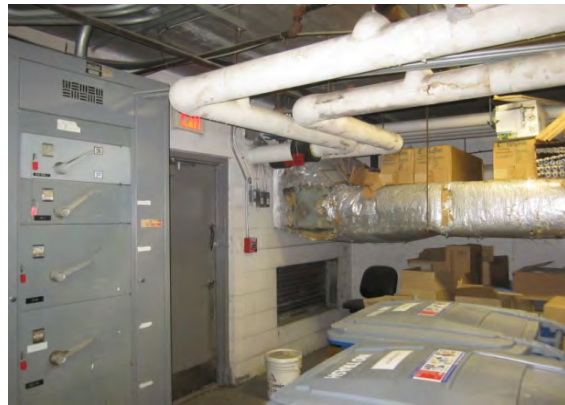
Photo 18: Insulated ducting and outdoor air louver
