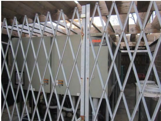
Photo 9: View of Trane chiller from outside
