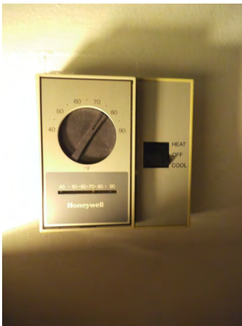
Photo 39: Thermostat for fan coil unit
