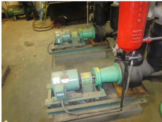
Photo 15: Hot water circulating pumps
