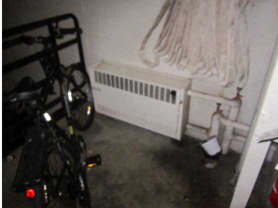
Photo 25: Unit heaters in stairwells
