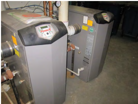
Photo 17: Hot water boilers recently installed
