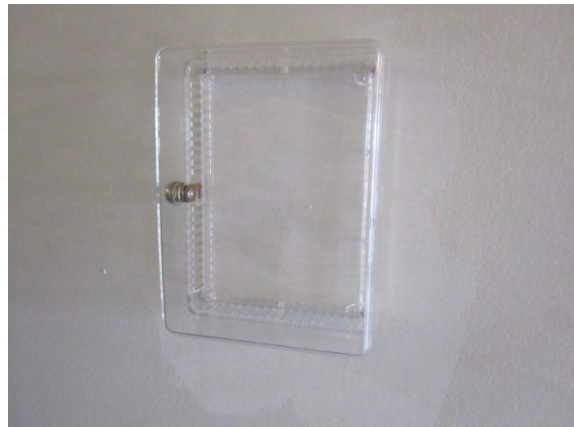
Photo 22: Casings for thermostats in hallways
