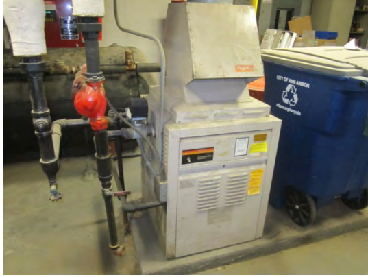
Photo 13: Older hot water boiler
