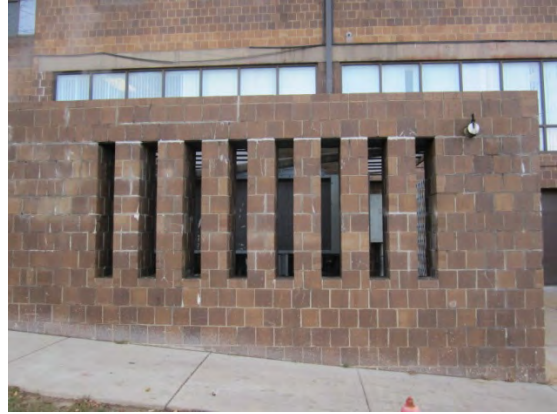
Photo 8: Housing for outdoor chiller
