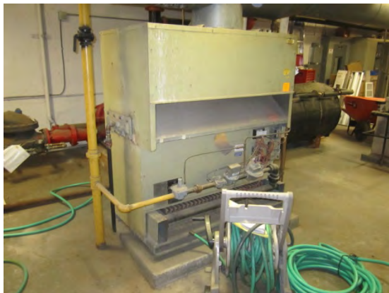
Photo 12: Domestic hot water boiler in basement
