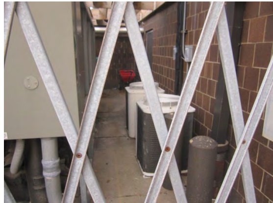
Photo 10: Additional condensing units near chiller
