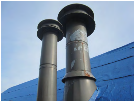
Photo 41: Central boiler vent stack on roof
