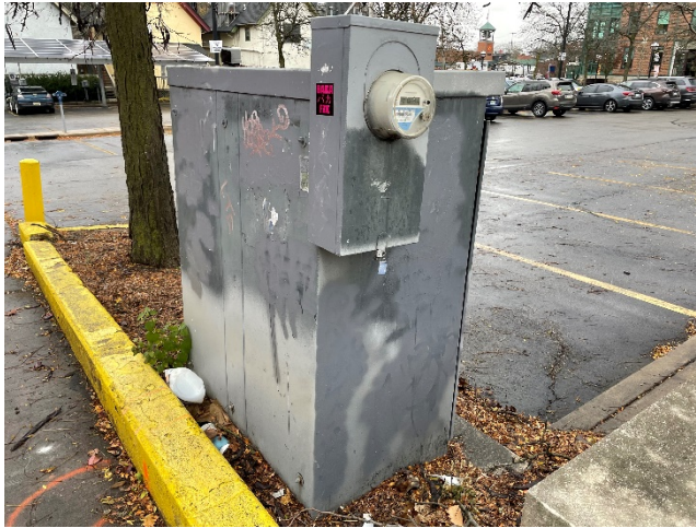
Photograph 4: Pad mounted transformer unit, southwest corner.
