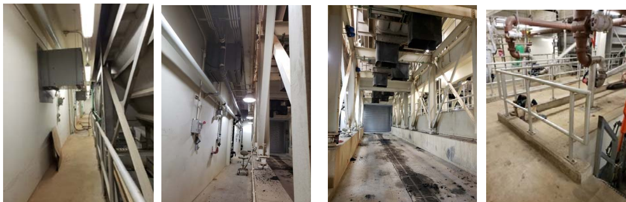
FIGURE 10: TRUCK LOADOUT HOPPERS AND TRUCK BAY
