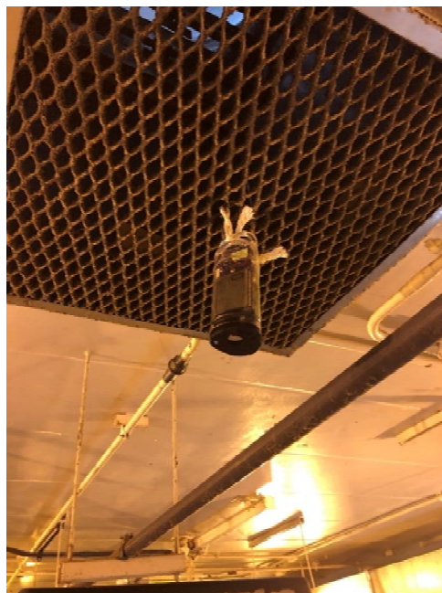
FIGURE 29: INLET OF SCREEN AND GRIT BUILDING EXHAUST FAN RF-25
