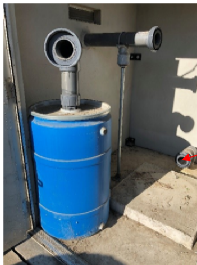
FIGURE 21: CARBON VENT FILTER INLET PIPE
