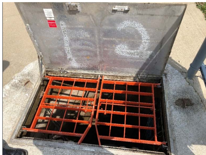
FIGURE 9: WCC FITNESS CENTER LIFT STATION
