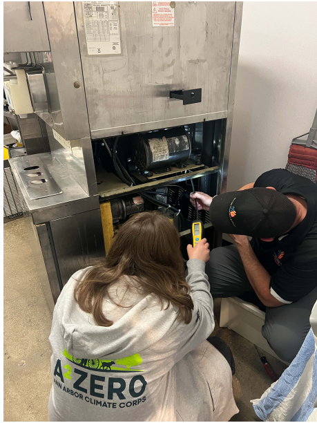
Refrigeration check at Blom Meadworks.
