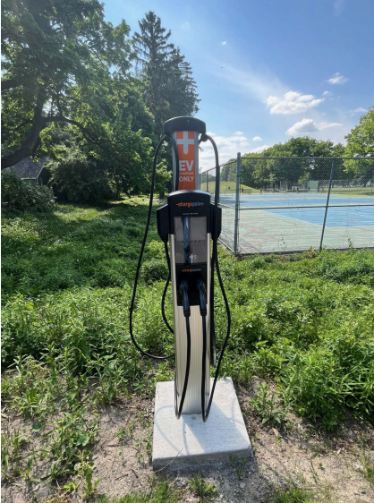
EV Charger at the Ann Arbor Senior Center.
