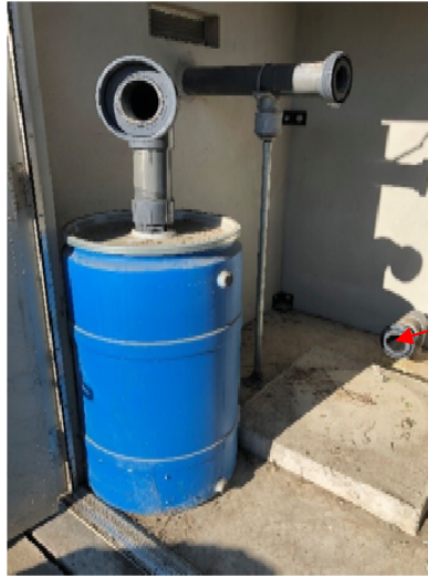
FIGURE 2: CARBON VENT FILTER INLET PIPE
