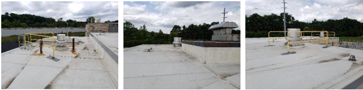
Figure 8 Roof Exhaust fans on the Screenings and Grit Building
