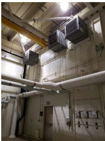
FIGURE 9: CENTRIFUGE ROOM EXHAUST FANS
