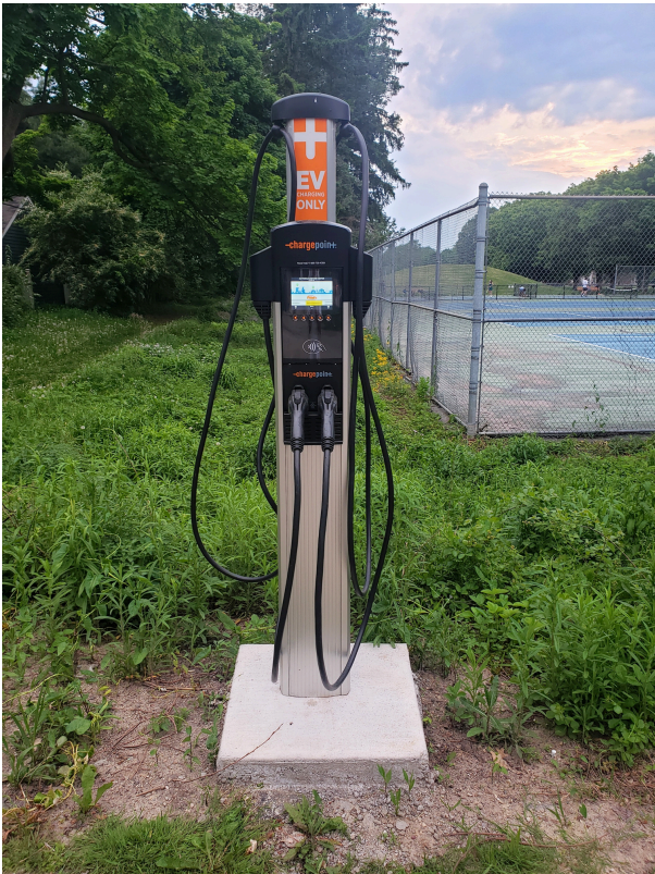
Electric vehicle charging station
