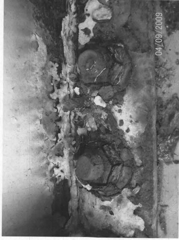
DETERIOATED ANCHOR NUT (SEE SHEET 2 FOR LOCATIONS. REPLACE IN ACCORDANCE WITH NOTES ON SHEET 2)
