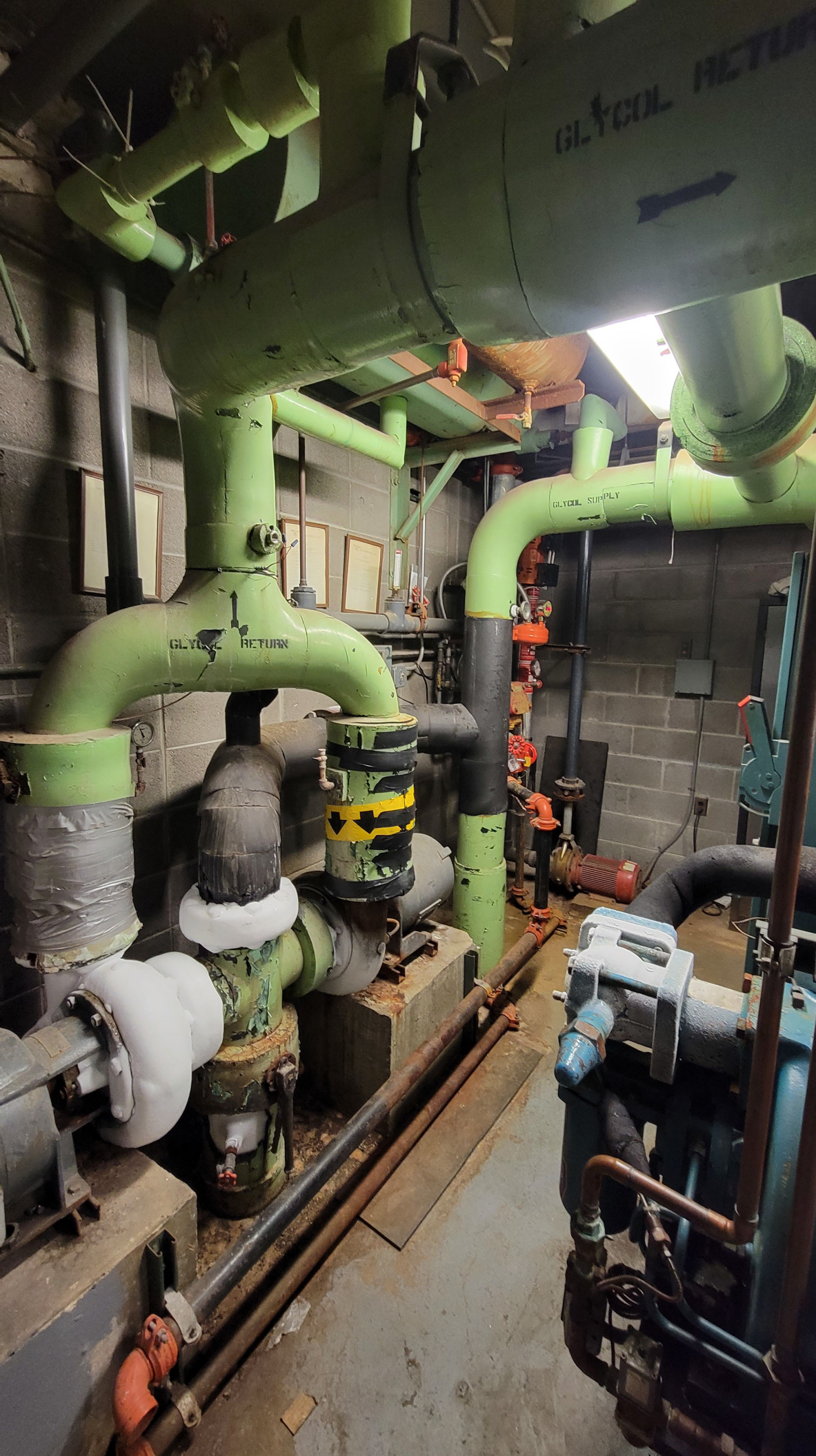
Glycol Return and Supply System
