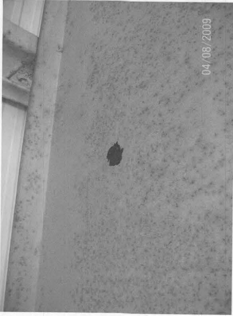
SAMPLE SURFACE RUST SPOTTING
