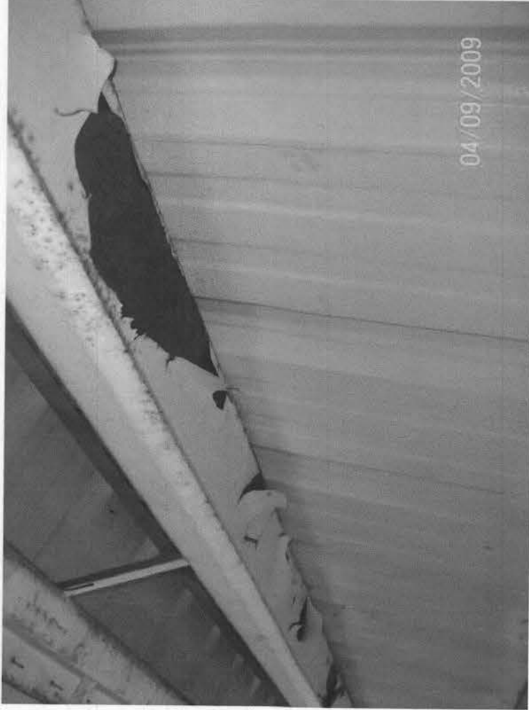
SAMPLE PAINT PEELING/FLAKING
