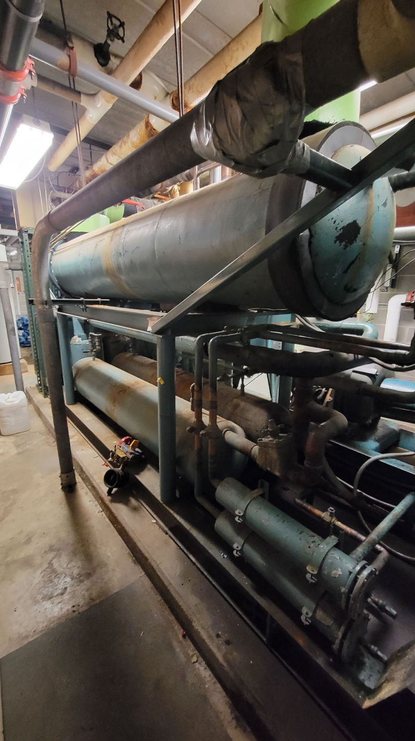
Rear view of Compressor 1
