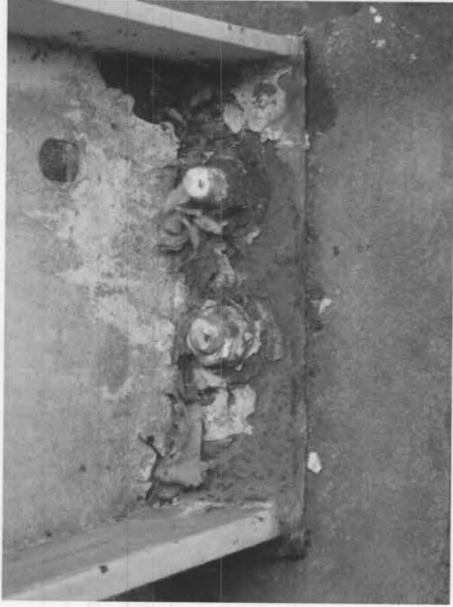
EX. SURFACE CONDITION (NOTE PRESENCE OF MILDEW)
