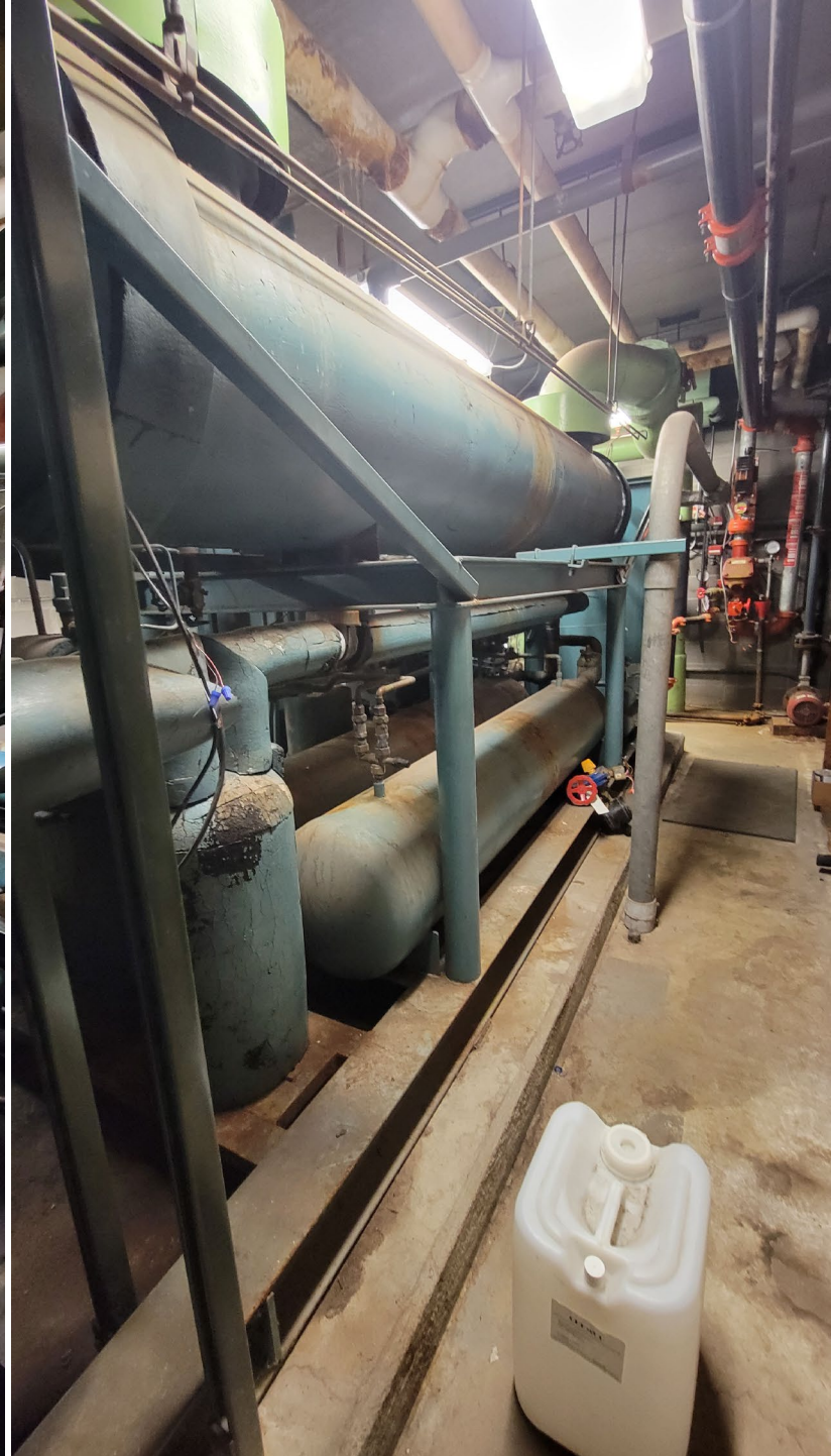
Rear view of Compressor 2
