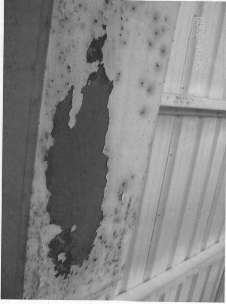
SAMPLE SURFACE RUST AREA
