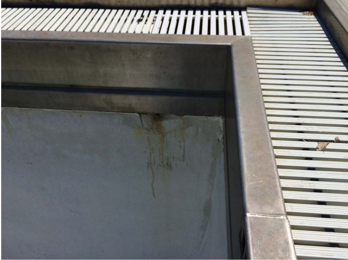
Spalling concrete beneath stainless steel gutter SW corner of deep pool
