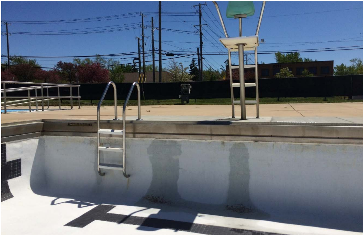
Leaking stainless steel gutter south wall east of deep pool
