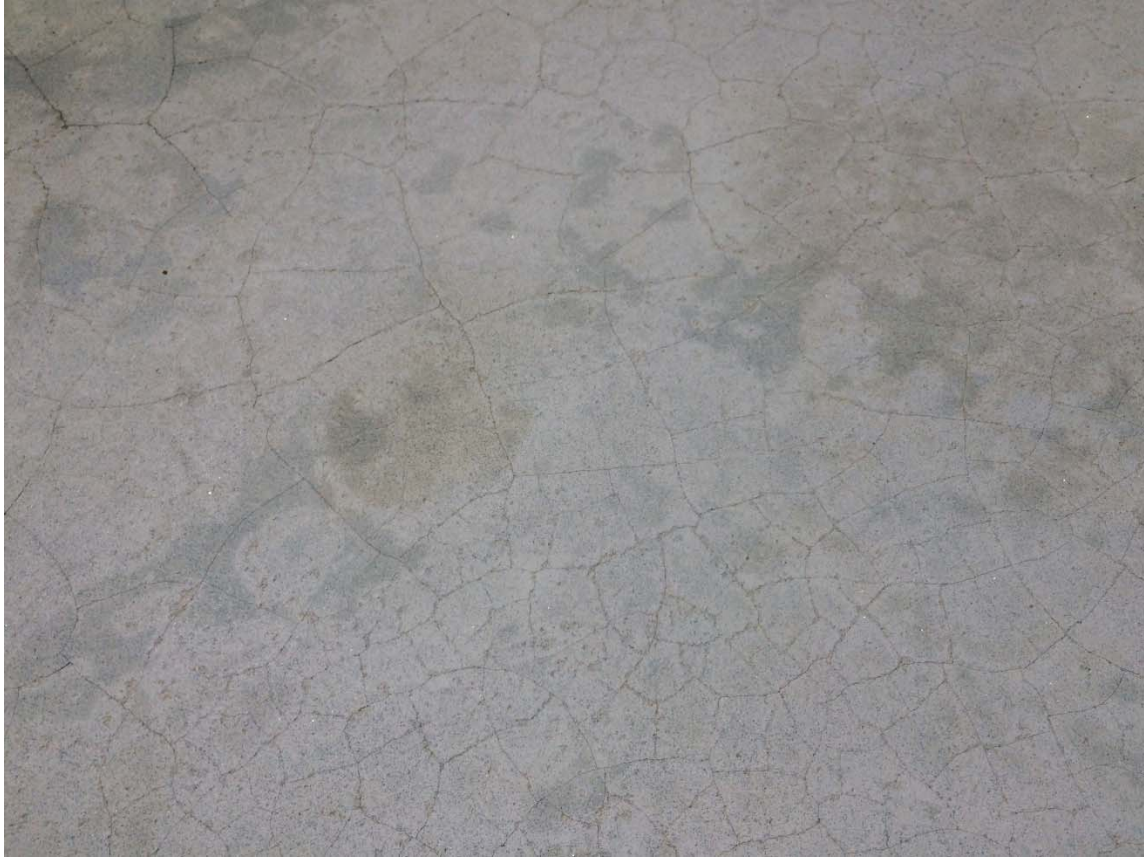
Delaminating Marcite in wading pool
