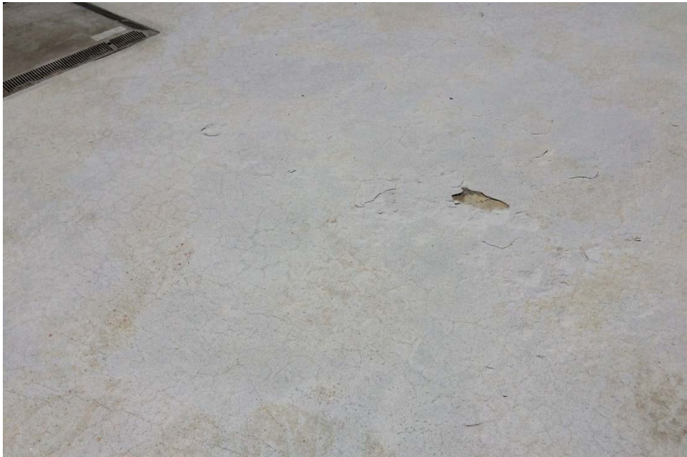
Delaminating Marcite in wading pool
