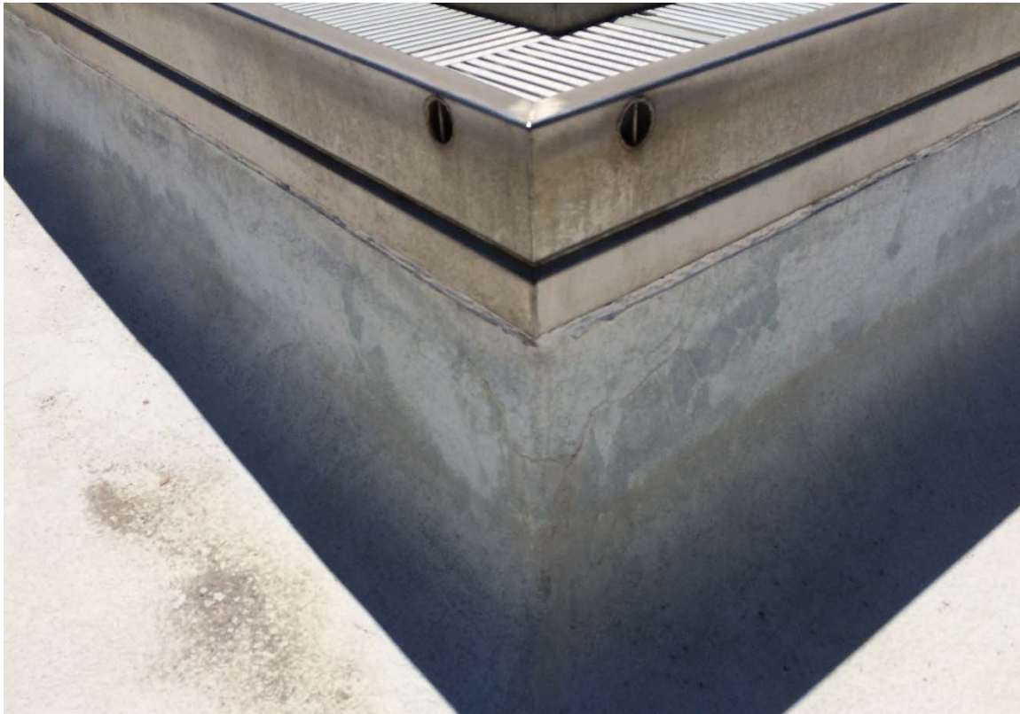
Delaminating Marcite in NW corner of wading pool
