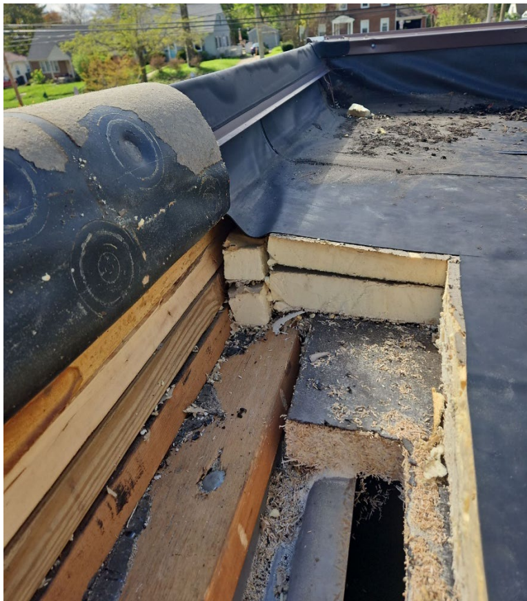
Cut Through at Leaning Parapet at Southeast Side of Lower Roof
