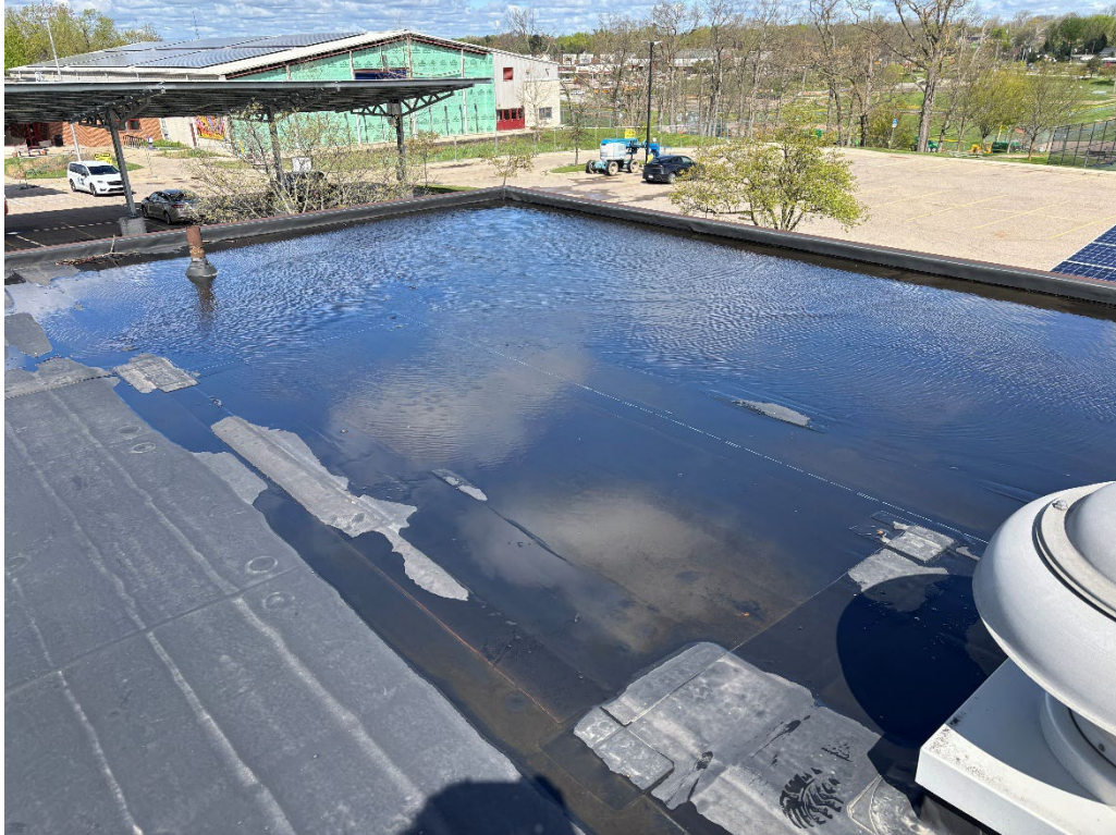
North Section of Upper Roof – Note Excessive Ponding, Must Be Addressed
