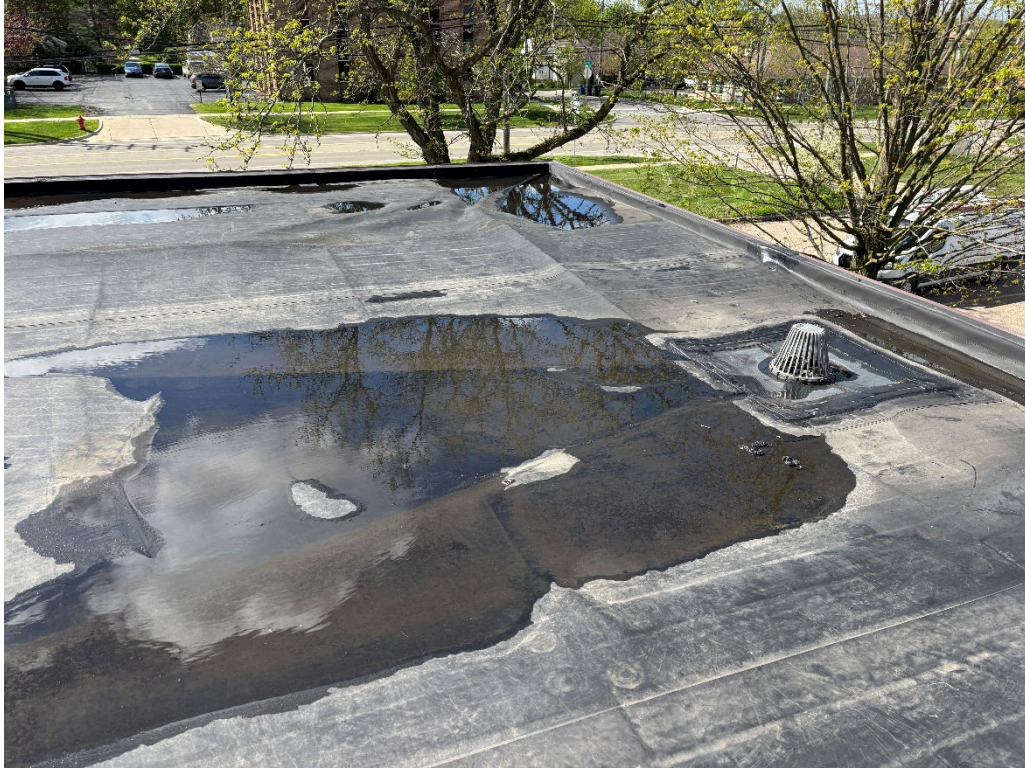
Southwest Corner of Upper Roof – Note Ponding Areas Due to Storm Damage
