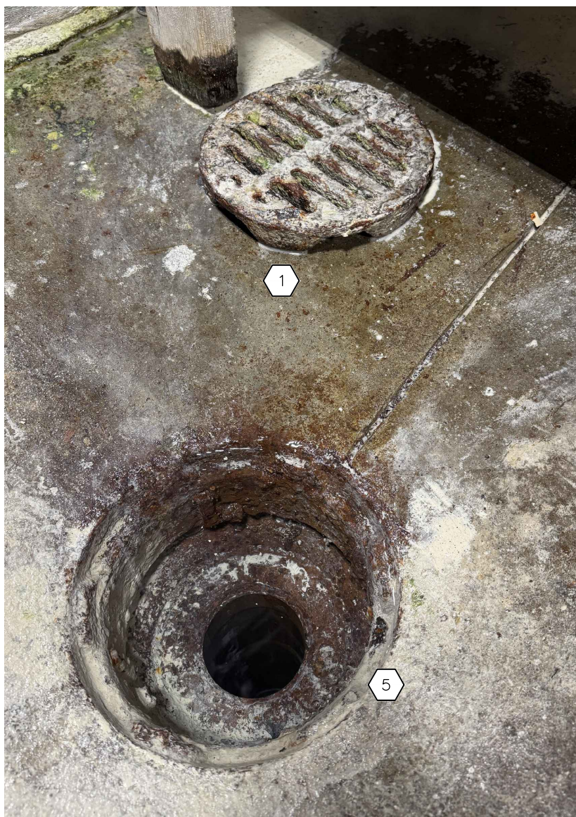
FLOOR DRAIN, TYPICAL PHOTO SCALE: NOT TO SCALE
