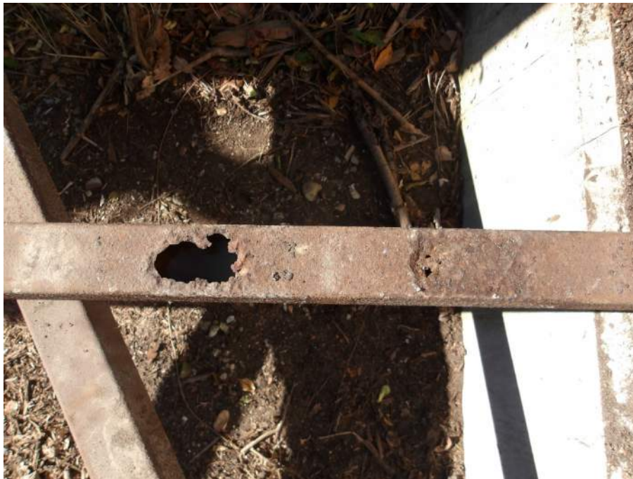
Photo 6 – Deficiencies in Steel Member 1W (Looking West)
