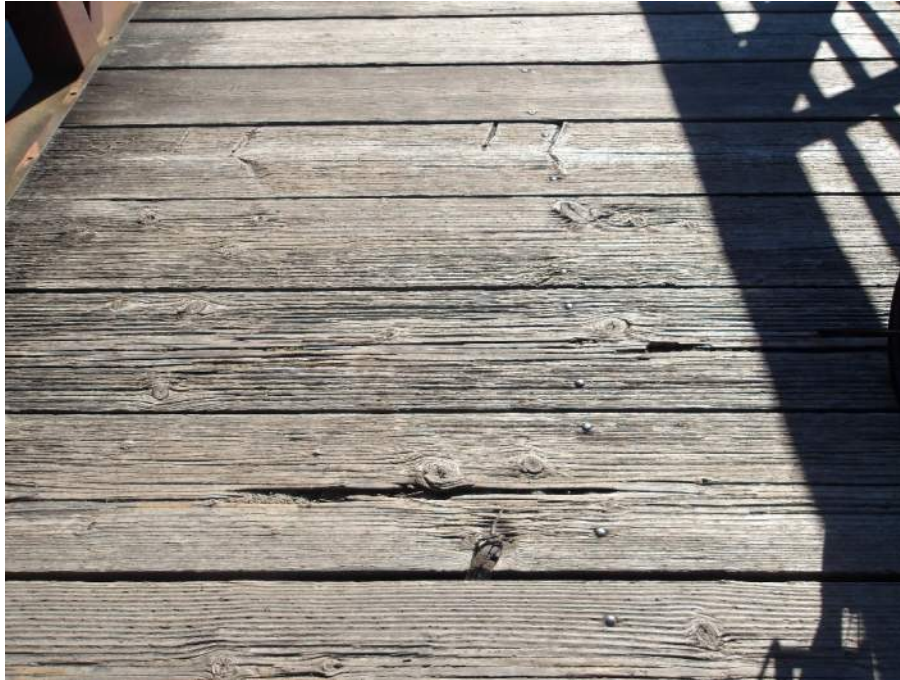
Photo 11 – Splintered / Delaminated Wood, 4 Boards (Looking South)
