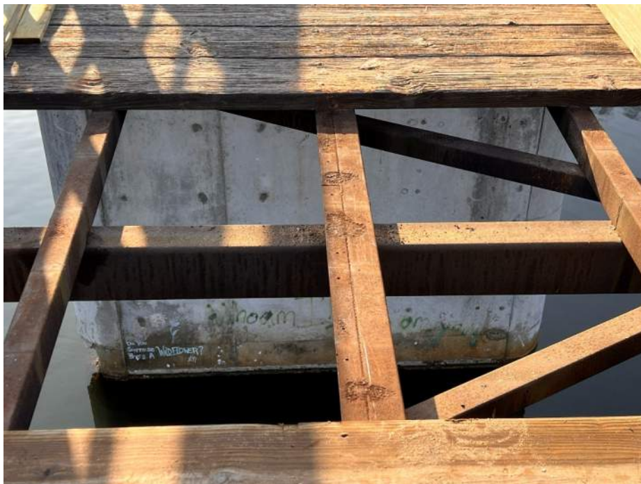
Photo 8 – Stringer Condition in Span 3 near Pier 2S (Looking South)
