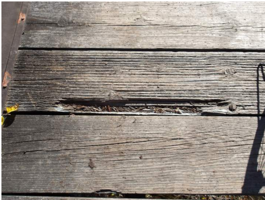
Photo 10 – Deck Deficiencies in Rotting Wood (Looking South)
