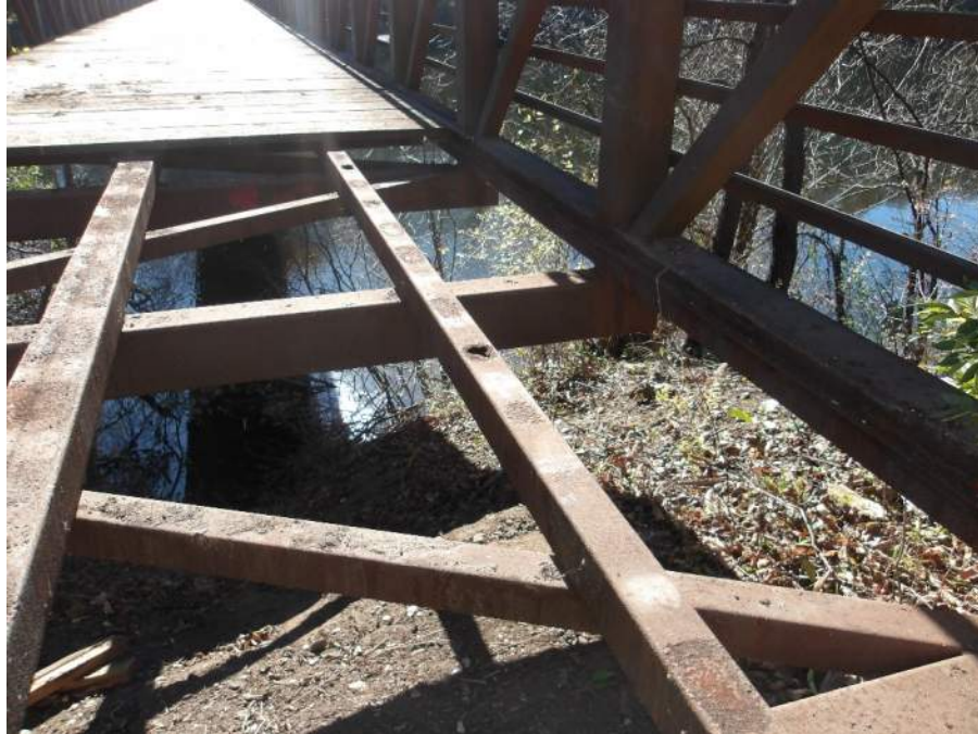
Photo 5 – Beam 1W Typical Section Loss and Heavy Pitting (Looking South)
