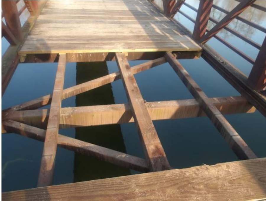
Photo 7 – Stringer Condition at Midspan of Span 3 (Looking South)
