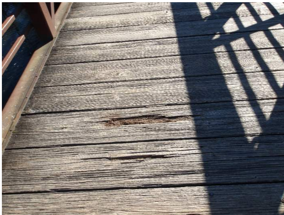
Photo 14 – Rotted Surface with Growth (Looking South)
