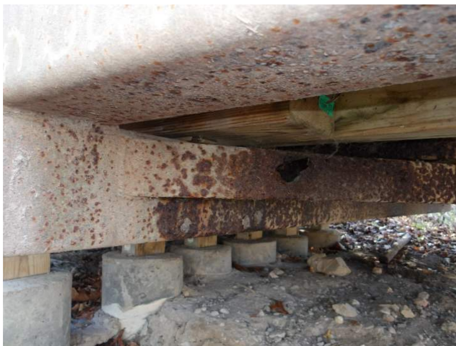
Photo 48 – 100% Section loss in cross frame (Looking Southwest)
