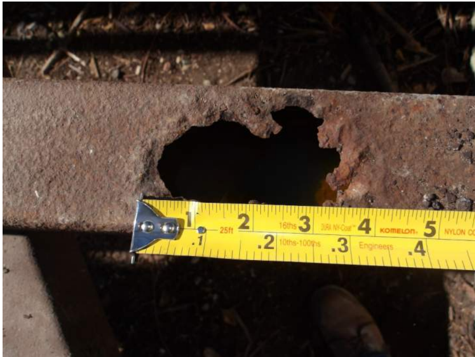
Photo 9 – Beam 1W Section Loss with Water in Beam (Looking West)
