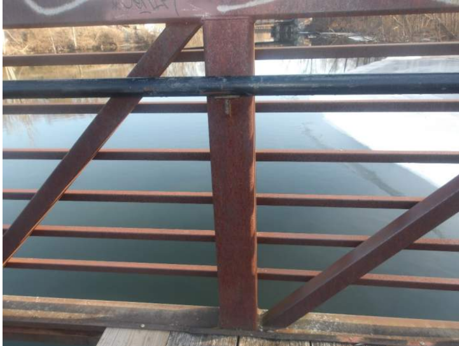
Photo 11 – Typical Corrosion on Truss Members (Looking East)
