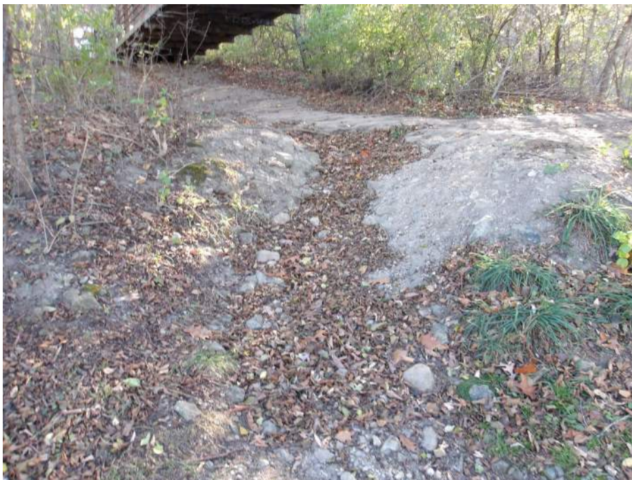
Photo 26 – Erosion Occurring under Span 1 in Southeast Quadrant Near Pier 1S (Looking Southwest)
