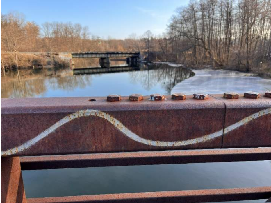
Photo 33 – Missing bolt in top of truss (Looking East)
