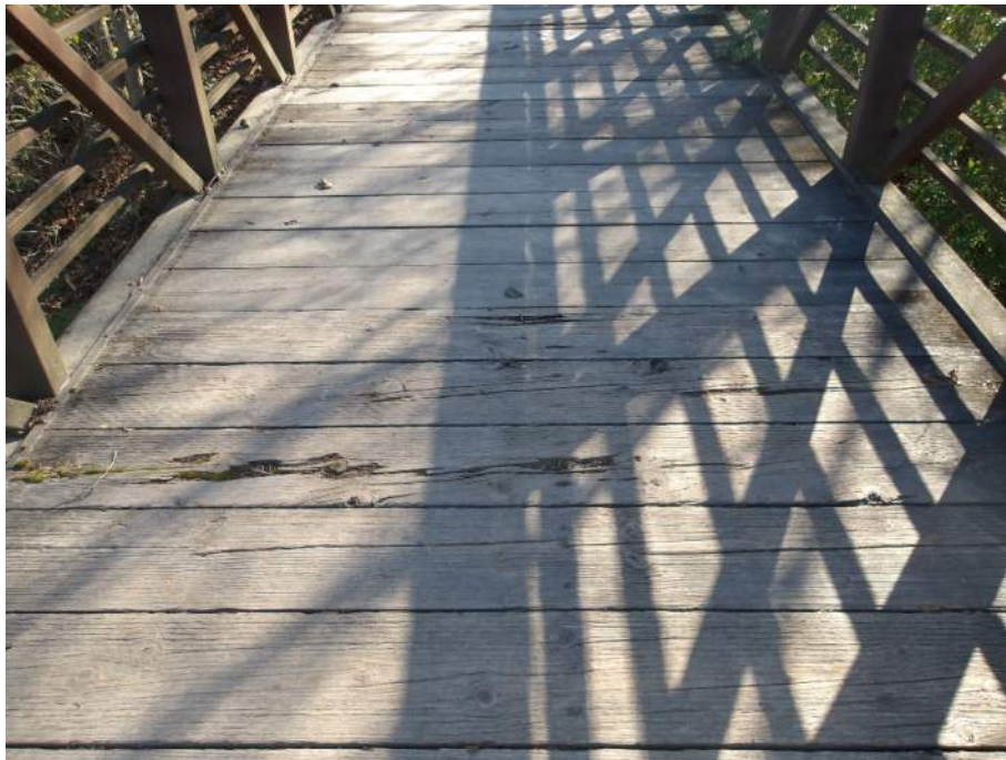
Photo 16 – Heavy Growth and Rot (Looking South)
