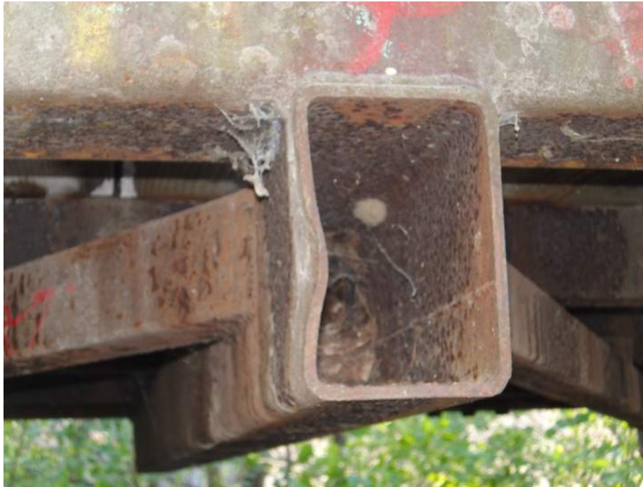
Photo 25 – Deformation in Floorbeam 8S, ½" Offset (Looking West)
