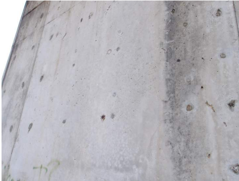
Photo 43 – Hairline crack on north face of Pier 2S (Looking South)
