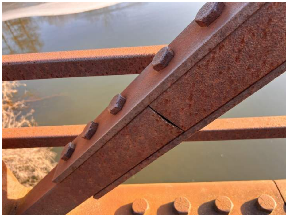
Photo 34 – Distortion in splice in East truss (Looking East)
