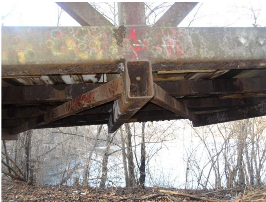
Photo 14 – Deformation in Floorbeam 8S, 1/2" Offset (Looking West)
