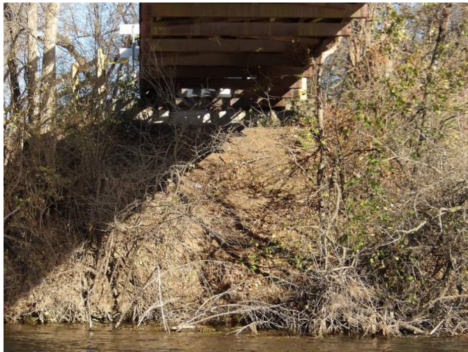
Photo 30 – Slope Erosion at North Embankment (Looking North)
