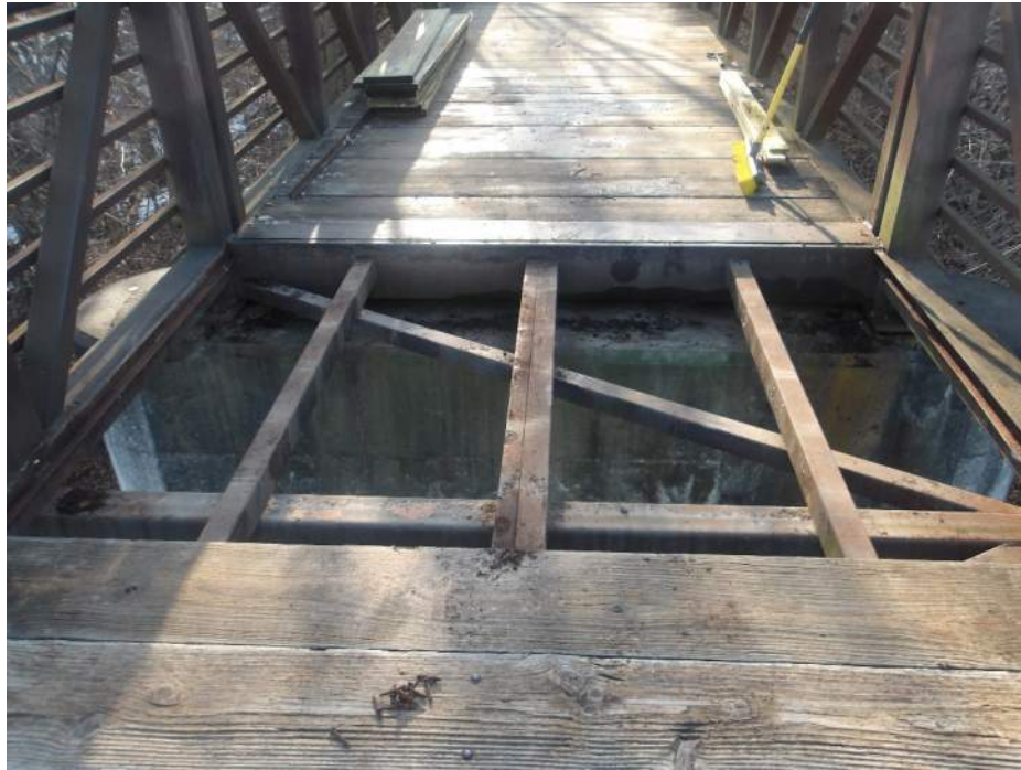
Photo 9 – Stringer Condition in Span 2 near Pier 1S (Looking South)
