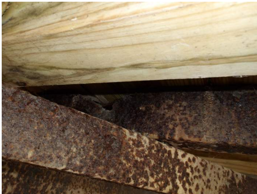
Photo 22 – 8"x2" area of 100% Section Loss, Top of Stringer 3W (Looking Southwest)
