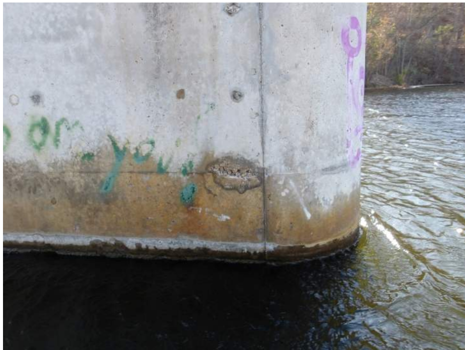
Photo 32 – Honeycombing on Pier 2S north face, 1sqft (Looking South)
