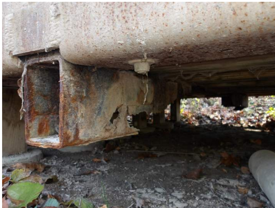
Photo 20 – 100% Section Loss, Floorbeam 2S (Looking Southwest)
