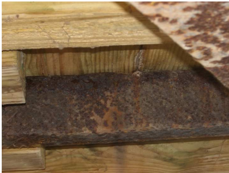
Photo 24 – 100% Section Loss 2" Long, Stringer 2W (Looking West)
