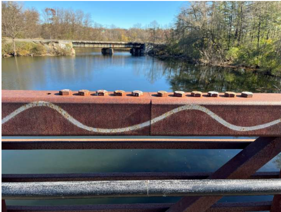
Photo 51 – Missing bolt in top of truss (Looking East)
