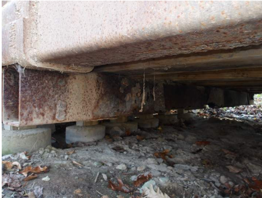
Photo 21 – 100% Section Loss at Bottom of Flange for 2/3 Length, Floorbeam 3S (Looking Southwest)
