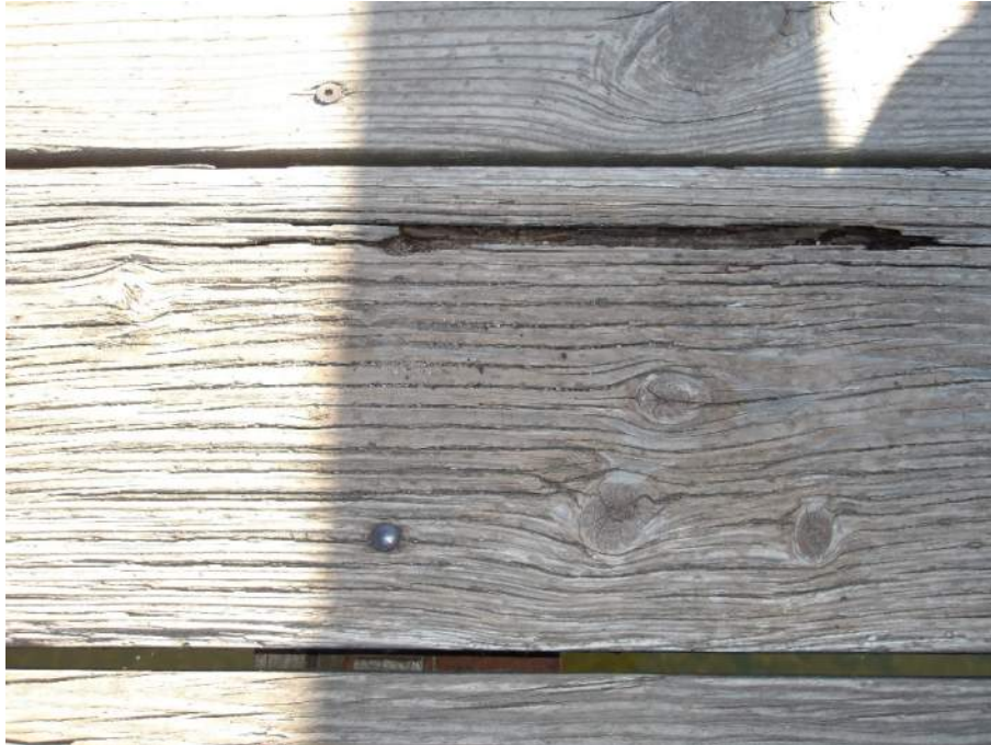
Photo 15 – Rotted Surface with Missing Rivets (Looking South)
