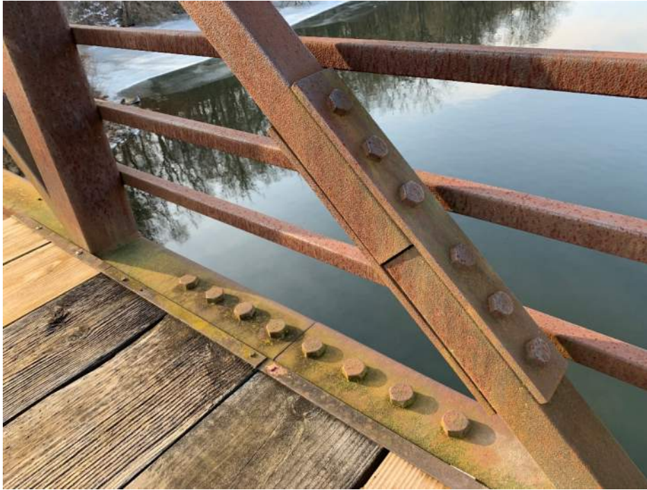
Photo 35 – Distortion in splice in West truss (Looking Southwest)
