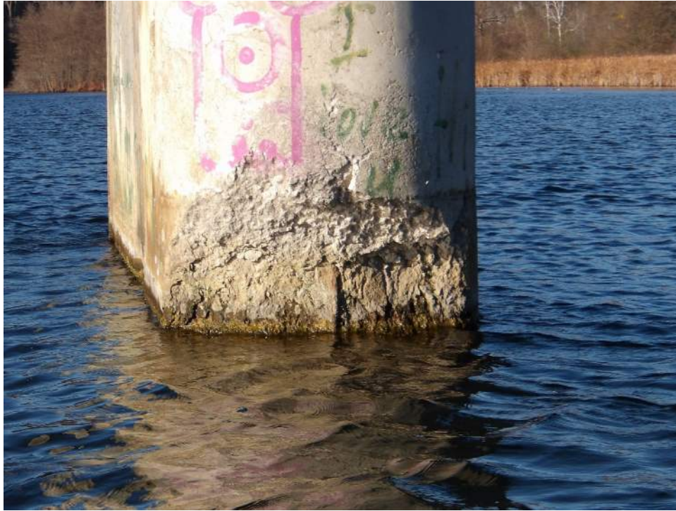
Photo 31 – Spall on Pier 2S (Looking West)
