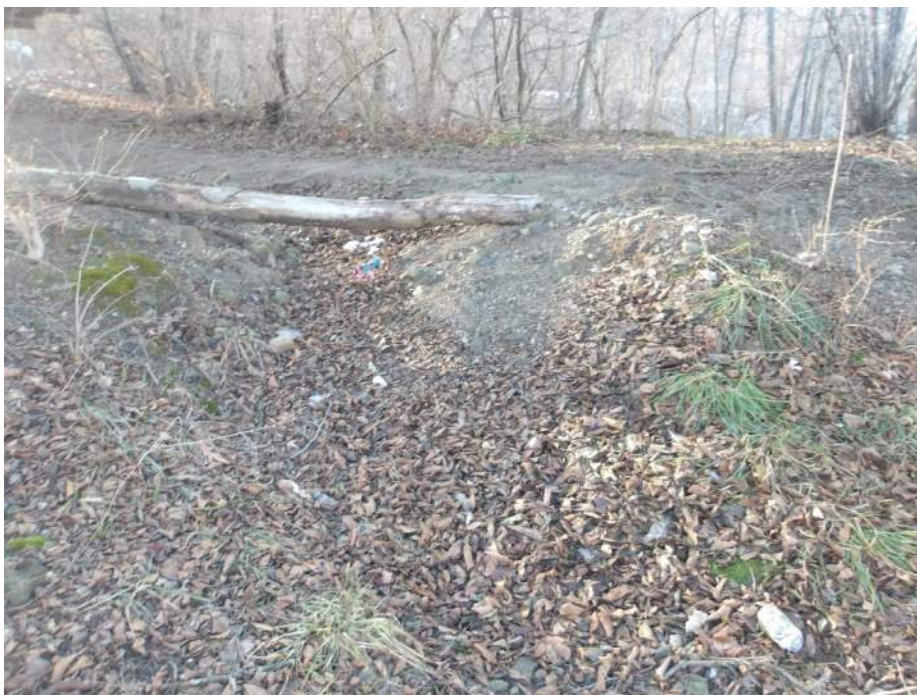
Photo 16 – Erosion Occurring under Span 1 in Southeast Quadrant Near Pier 1S (Looking Southwest)
