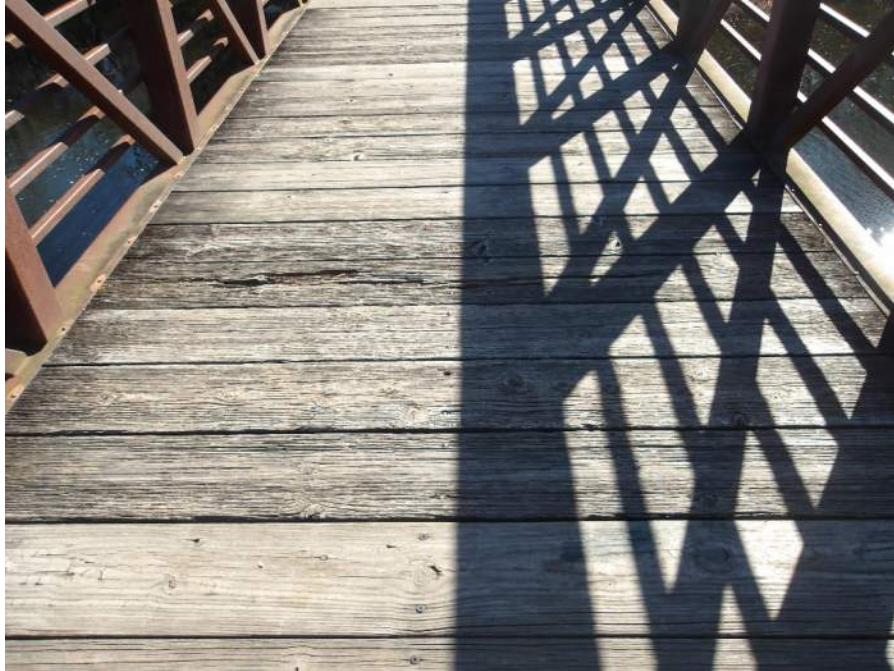
Photo 13 – Splintered / Delaminated Wood, 17 Boards (Looking South)
