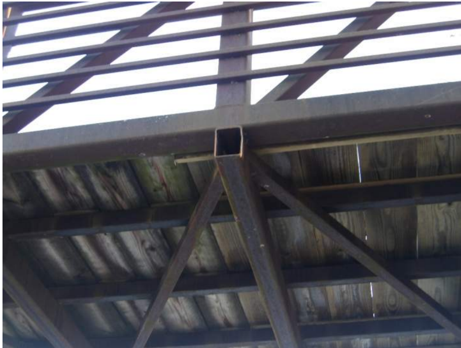
Photo 15 – Deformation in Span 2 Floorbeam near Pier 1, 1/2" Offset (Looking East)
