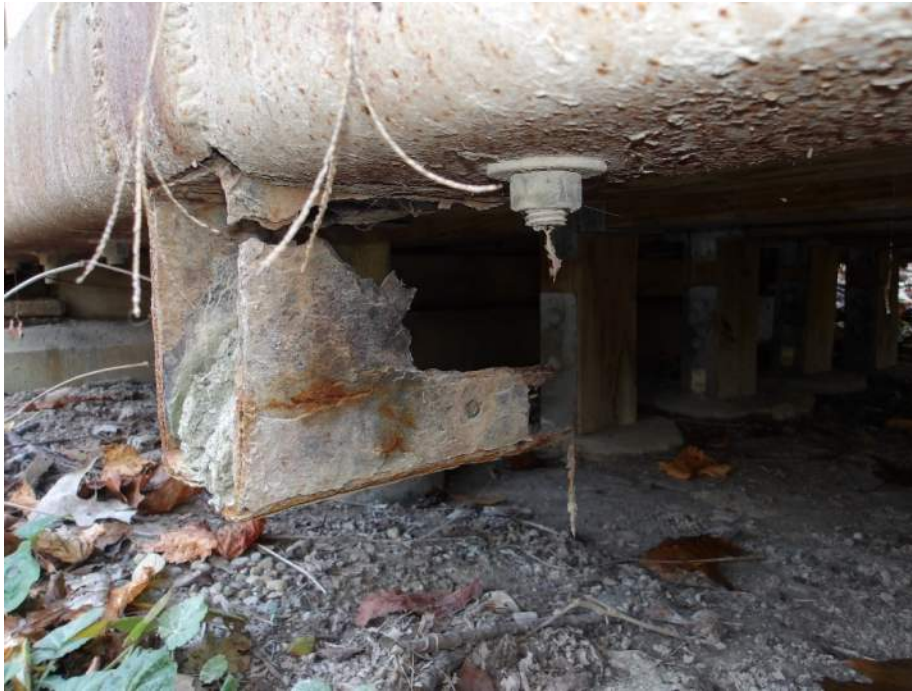
Photo 19 – 100% Section Loss, Floorbeam 1S (Looking Southwest)
