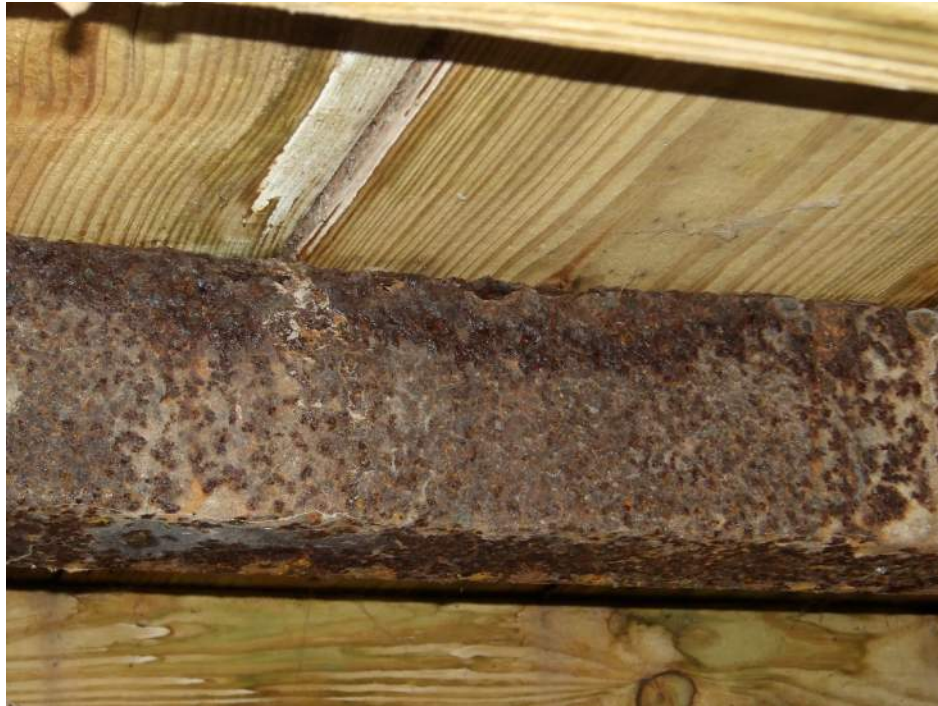
Photo 23 – 6"x0.5" area of 100% Section Loss, Top of Stringer 2W (Looking West)
