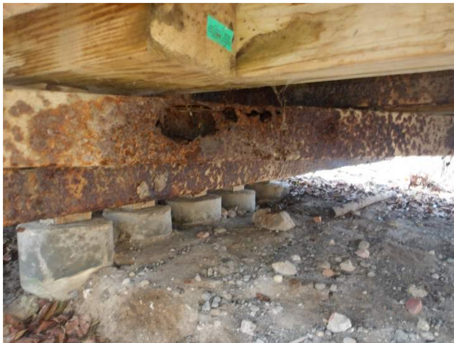
Photo 30 – 100% section loss in cross frame (Looking Southwest)
