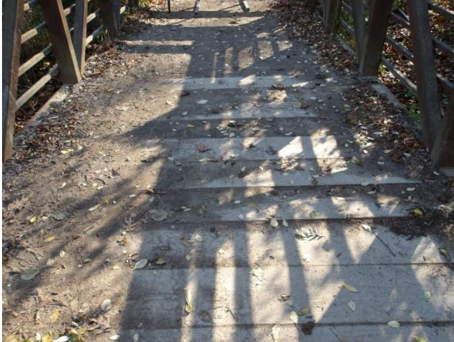
Photo 17 – Heavy Debris on Shoulders and Last 10ft of South End. Three Uneven Boards on West Barrier (Looking South)
