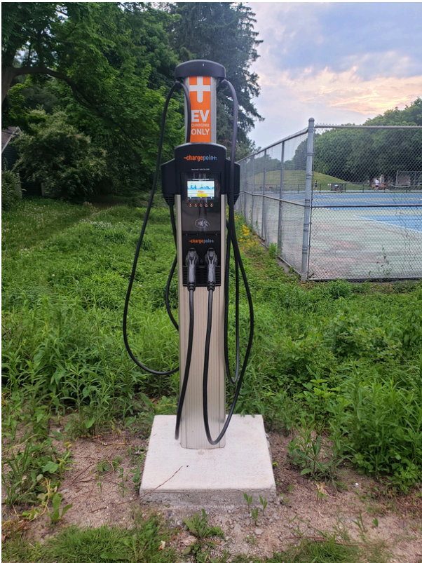
Electric vehicle charging station
