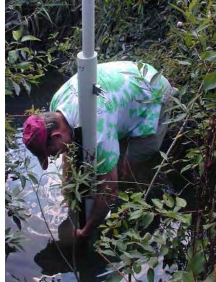
Figure 3.4 A volunteer installs a transducer at the Meadows study site.
