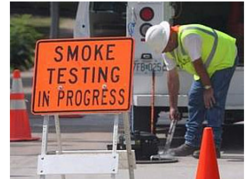
Field crews blow a non-toxic mist into the sanitary sewer system. The mist travels through the sewer lines, revealing problems in the system.
