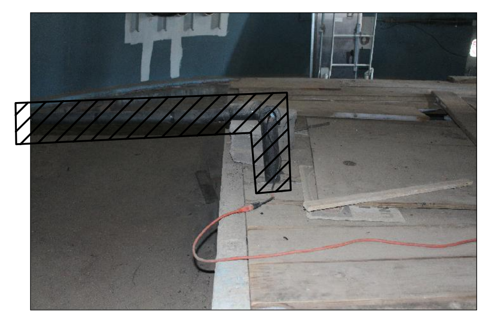
3 PHOTO HEAT TRACE & SUMP DISCHARGE SCALE: NA
