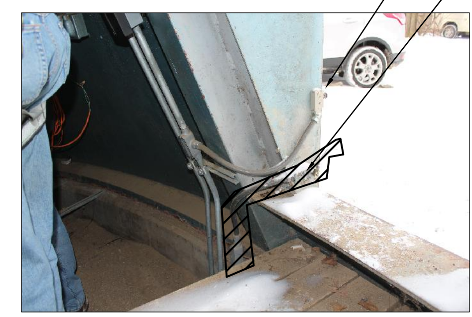
2 PHOTO DOOR CONTACT (SWITCH) SCALE: NA
