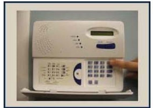
Alarm key pad
