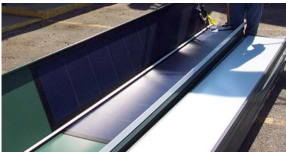
Farmers Market roof sections with solar panels.
