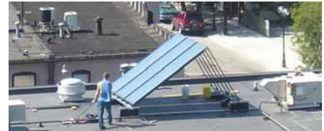
Solar hot water panels on Ann Arbor Fire Station #1
