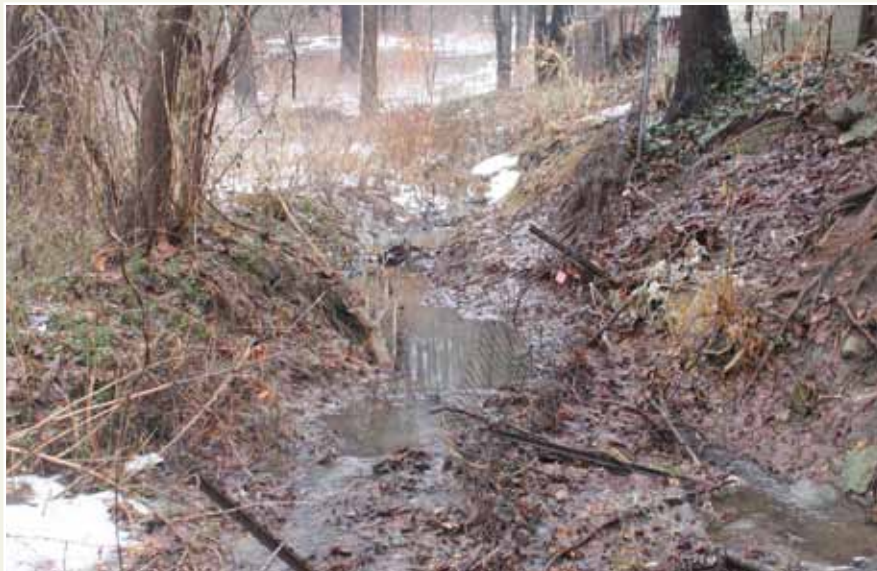
channel erosion prior to rehabilitation
