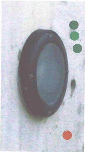
Wall-Mounted Stair Light
