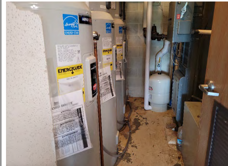
Photo 13. View of the utility room
