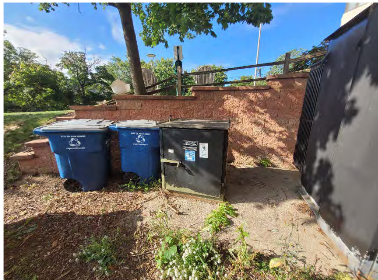
Photo 15. View of the pad-mounted transformer
