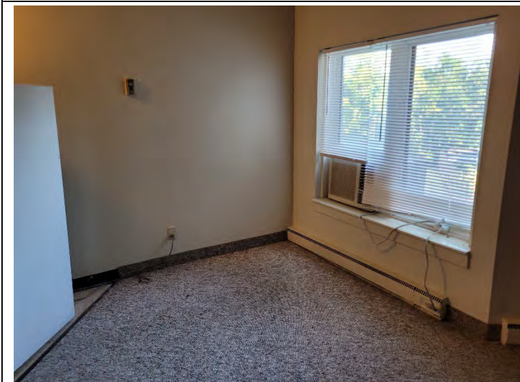
Photo 11. View of a typical living area with AC unit and electric baseboard heat
