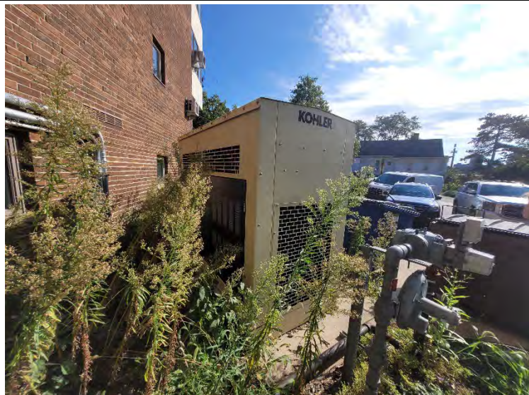
Photo 14. View of the natural-gas-powered emergency generator
