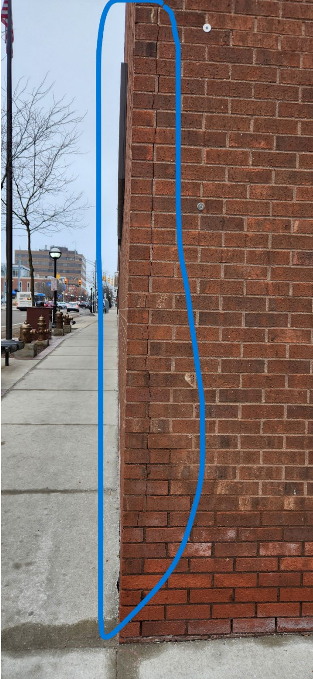
(above) Crack 2 corner of Ann and Fifth
