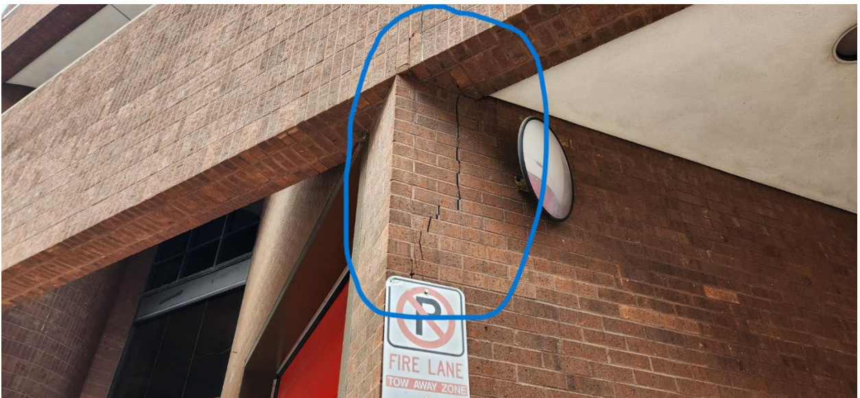
(above) Crack 1 by south entrance
