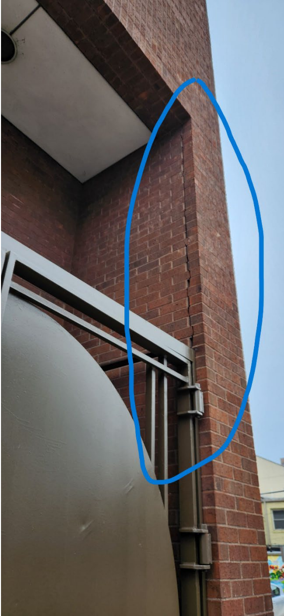
(above) Crack 3 on northwest side corner of building by Hands-on Museum
