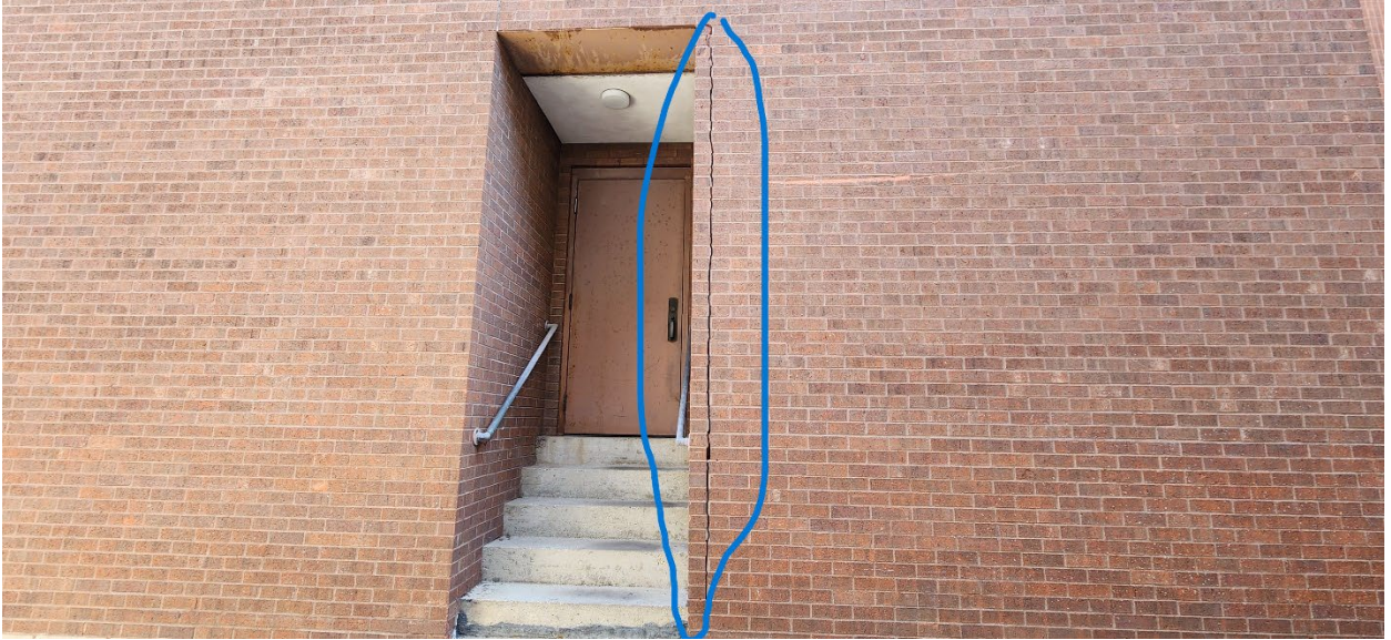
(above) Crack 4 west side of building by Hands-on Museum
